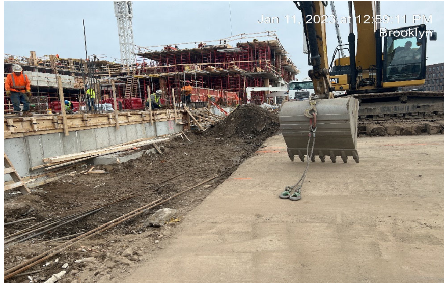
Photograph 1 - Civetta stockpiling remaining soil in WC-11 to be exported, view facing east.
