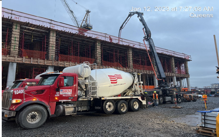
Photograph 1 - Broadway Concrete pouring concrete in forms of super structure, view facing northeast.
