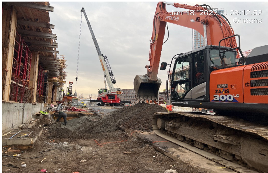
Photograph 2 - Dubner Landscaping excavating for sewer pipe adjacent to road in WC-19, view facing west.
