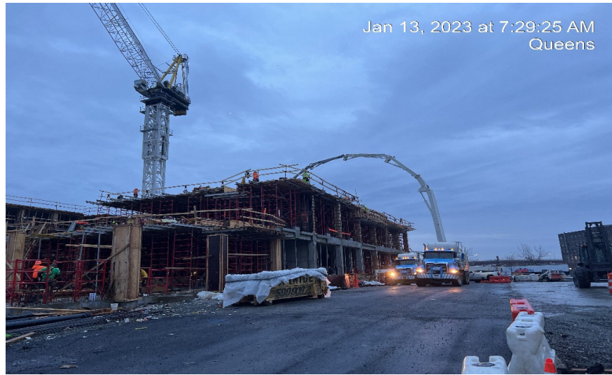
Photograph 1 - Broadway Concrete pouring concrete in forms of super structure, view facing east.
