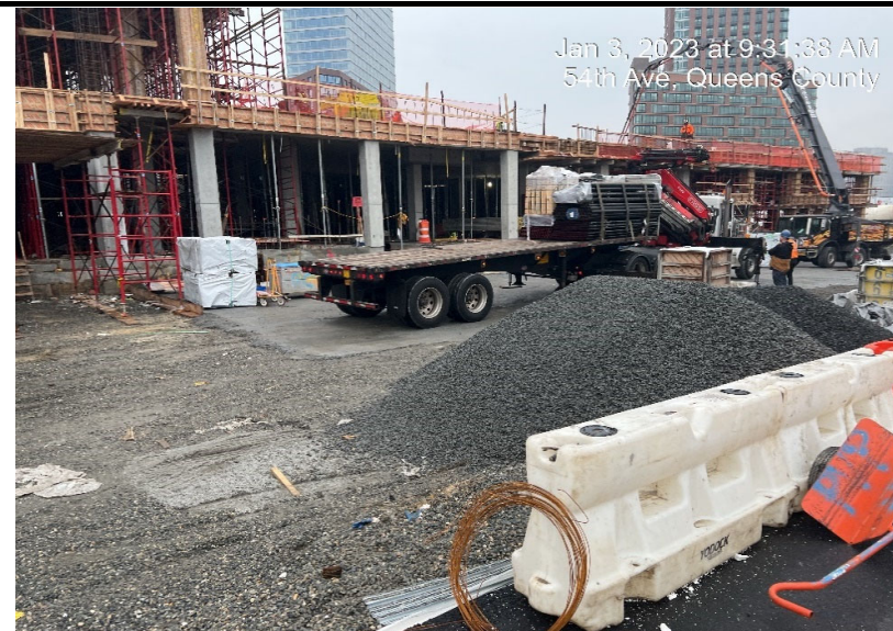
Photograph 3 - CCJV imports one load of No. 2 stone from Impact Stone Industries in Haledon, NJ, view facing southwest.
