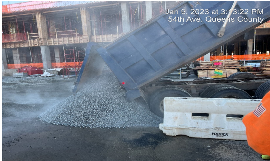
Photograph 1 - Civetta imports No. 2 stone from Impact Stone Industries, Haledon, NJ to WC-19, view facing south.
