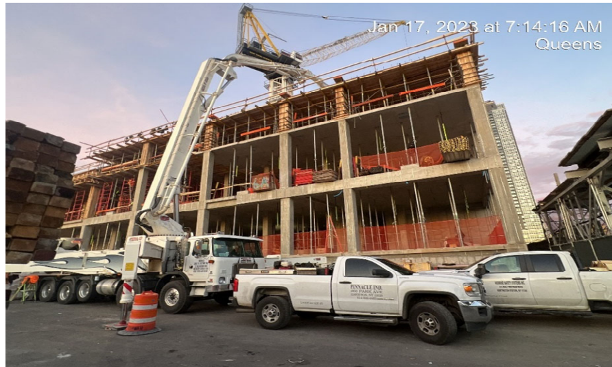
Photograph 3 - Broadway Concrete pouring concrete in forms of super structure, view facing west.
