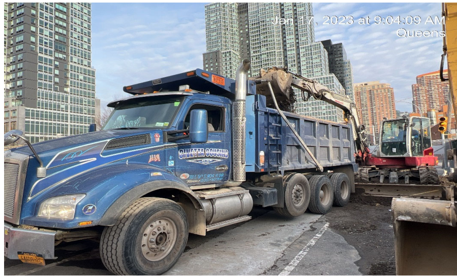
Photograph 1 - CCJV exporting 1 load from WC-01 (3.5-7') to Bayshore Management LLC, view facing north.
