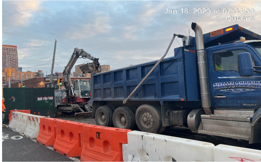
Photograph 1 - CCJV exporting 1 load from WC-01 (3.5-7') to Bayshore Management LLC, view facing north.
