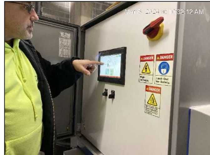
Photograph 2: SVE control panel.
