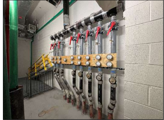
Photograph 2: View of the eastern SSDS manifold in sewer room.
