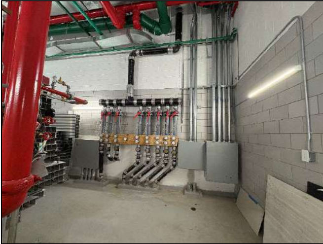
Photograph 1: View of the western SSDS Manifold in western compactor room.
