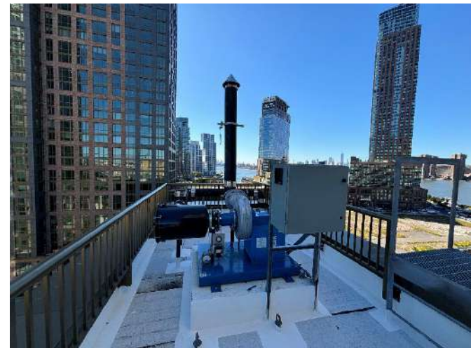
Photograph 4: View of SSDS effluent stack on 8 th floor.
