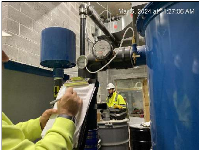
Photograph 1: SVE System startup.
