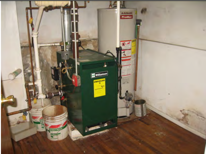
1-STORY DWELLING BOILER
