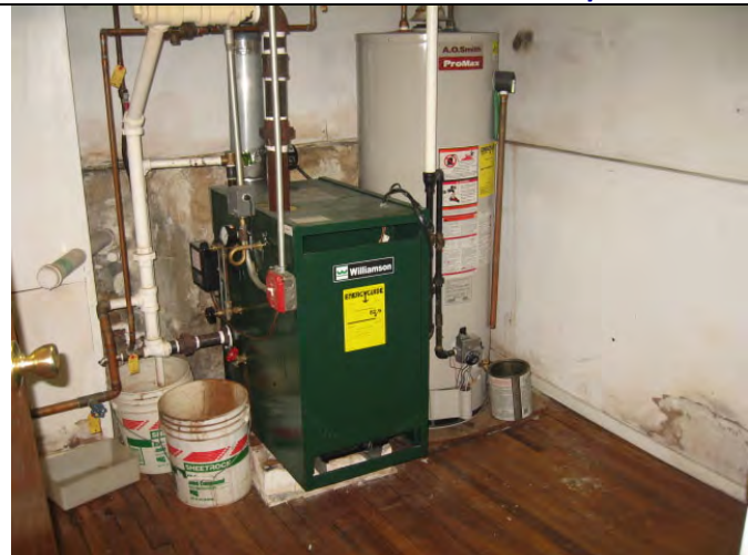
1-STORY DWELLING BOILER
