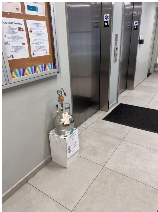
Photograph No. 9: View of IA-8 located proximally to the eastern building elevator.
