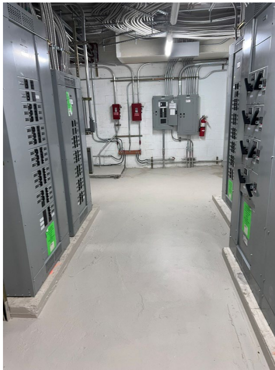
Photograph No. 13: View of electrical room.
