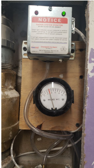
19. Typical alarm and gauge for RP-3 and RP-4
