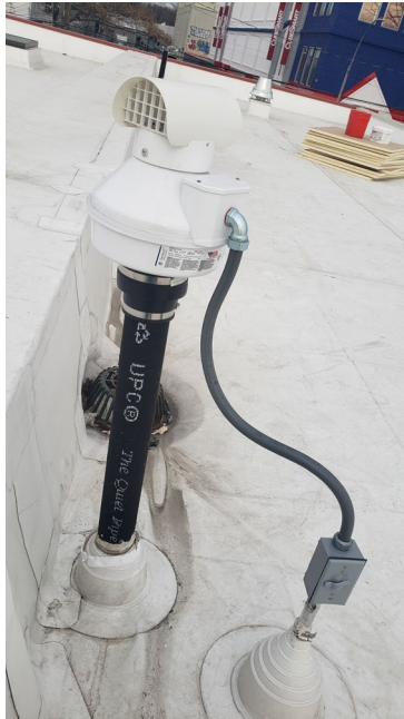
21. Typical rooftop mounted fan construction (RP-1 and RP-2)
