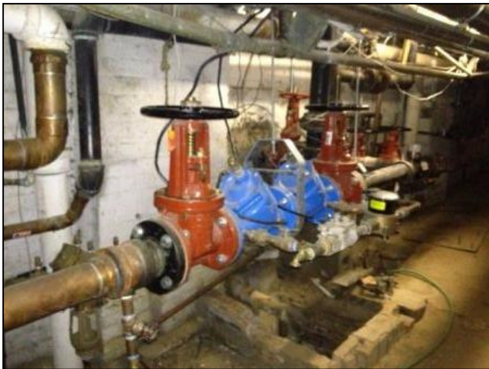
The Site utilizes municipal water for fire protection and other purposes.
