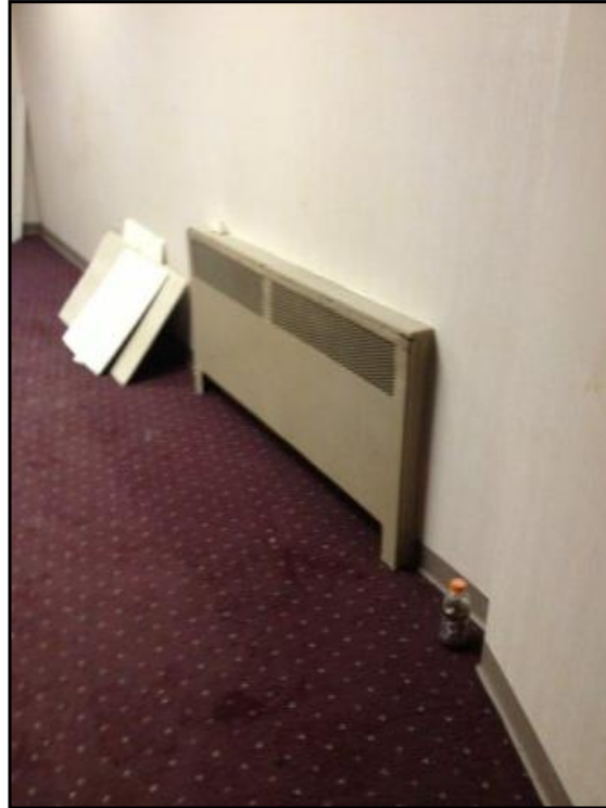
Steam heat is distributed throughout the building by radiators.
