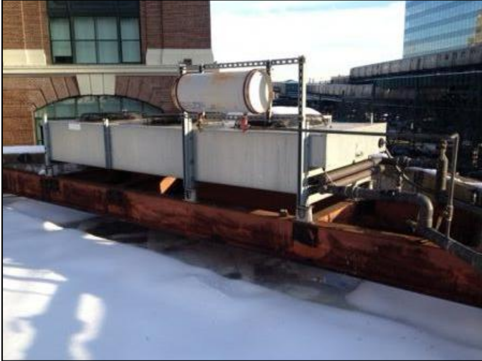
Electrical powered units on the roof provide air conditioning to the second floor offices and some of the commercial ground floor tenant spaces.
