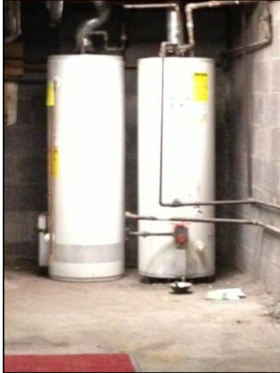
Hot water is provided to the building occupants by individual electric hot water heaters.
