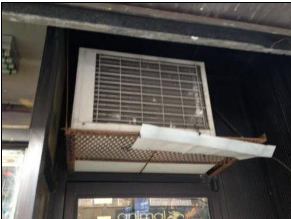
Window-mounted units provide air conditioning to some ground floor tenant spaces. remaining occupants of the Site receive air conditioning from window mounted units.
