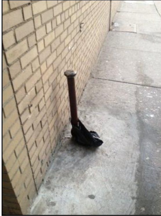
The vent pipe for the UST can be seen along the west exterior wall of the 2-story building fronting Crescent Street.
