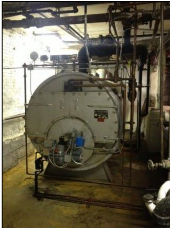
An oil-fired boiler in the basement produces steam heat to the building.
