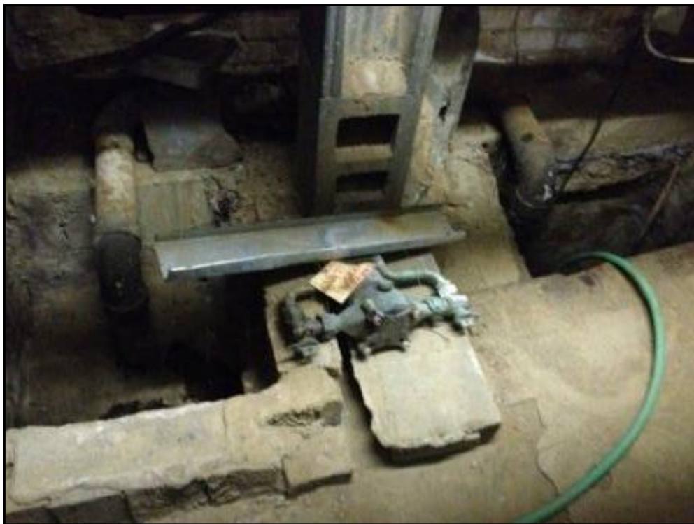
Waste generated at the Site is conveyed to the City sewer system.
