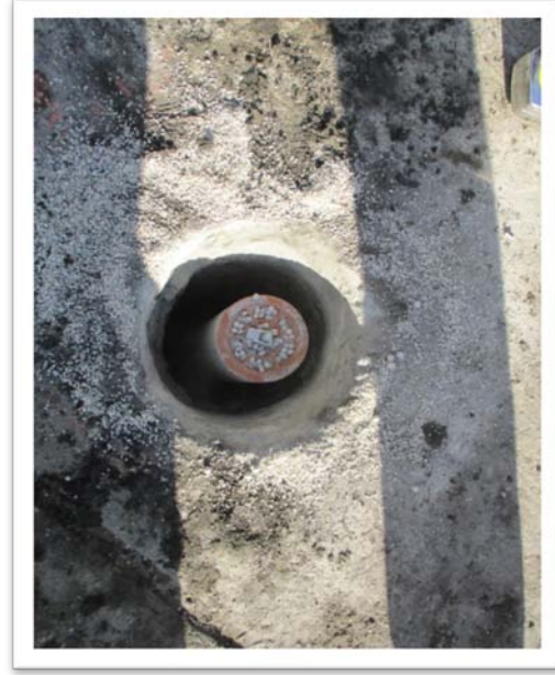
6. Installed Monitoring Well
