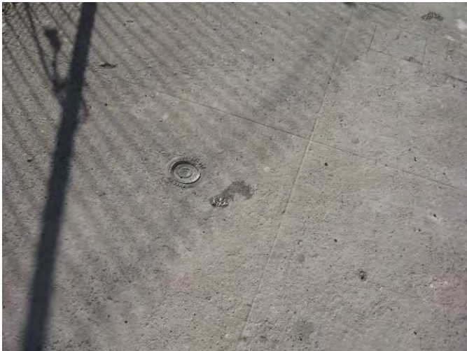
Typical fuel oil fill port at 94 th Ave. sidewalk
