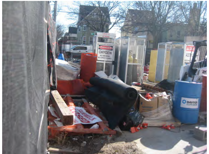
Compressed oxygen and acetylene storage
