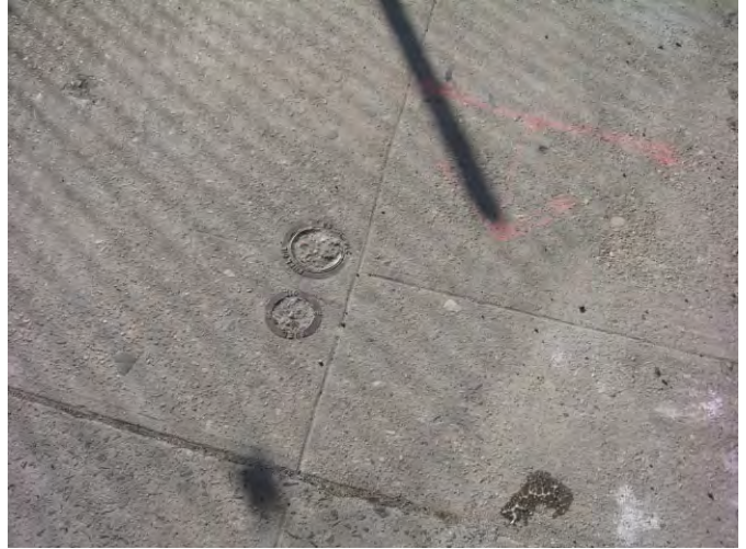
Typical fuel oil fill ports at 94 th Ave. sidewalk
