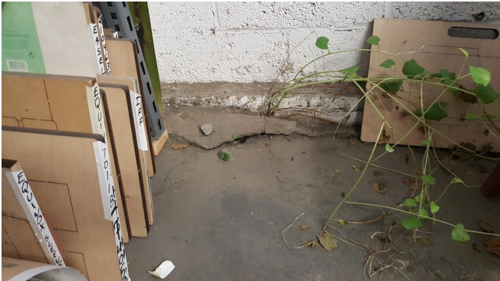
Photograph No. 6: View of western exterior wall conditions in northern warehouse area
