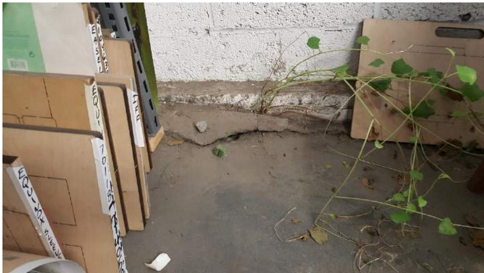
Photograph No. 6: View of western exterior wall conditions in northern warehouse area
