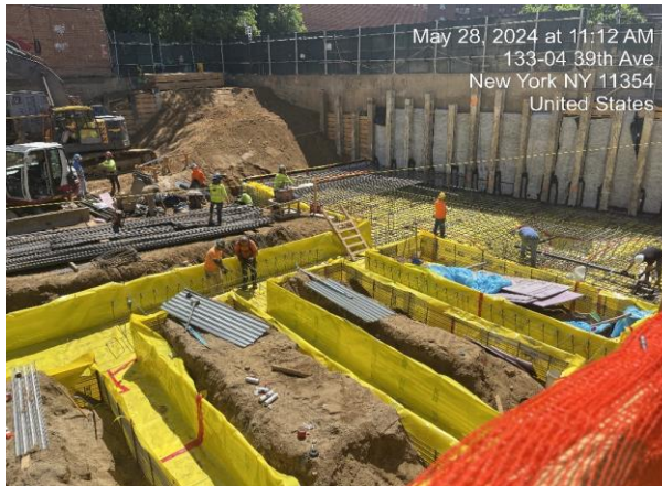
Photograph 2 - Installing 20-mil Stego Wrap vapor barrier and rebar in the southwestern portion of Site.
