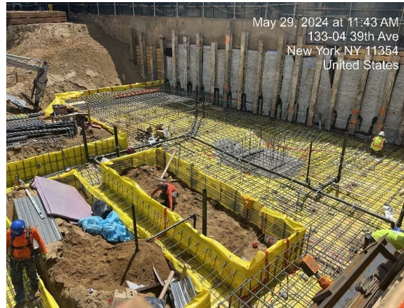
Photograph 2 - Contractor installed rebar in the southwestern portion of the Site as part of the foundation construction.
