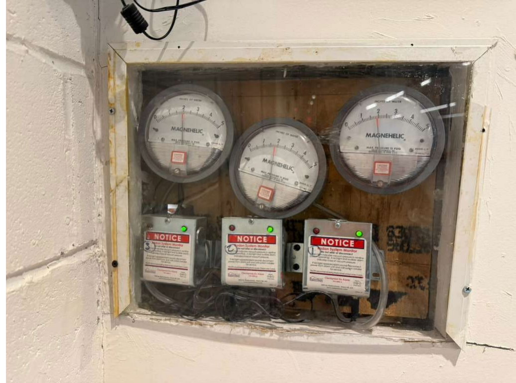
Dwyer magnehelic gauges and alarms at SSDS Pit 1 to Pit 3
