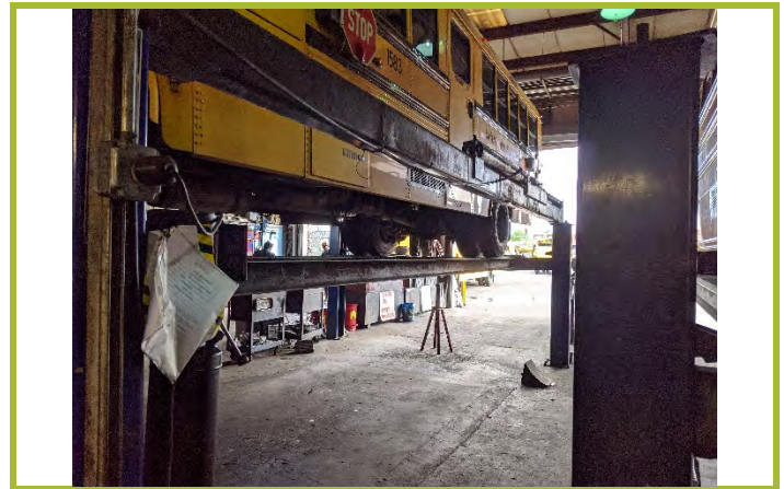
Photo #4: Typical aboveground hydraulic lift in Maintenance Garage.
