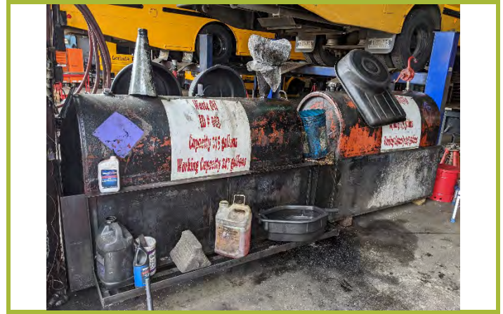
Photo #8: Two 275-gallon aboveground storage tanks (ASTs) located in the Maintenance Garage. Petroleum staining observed.
