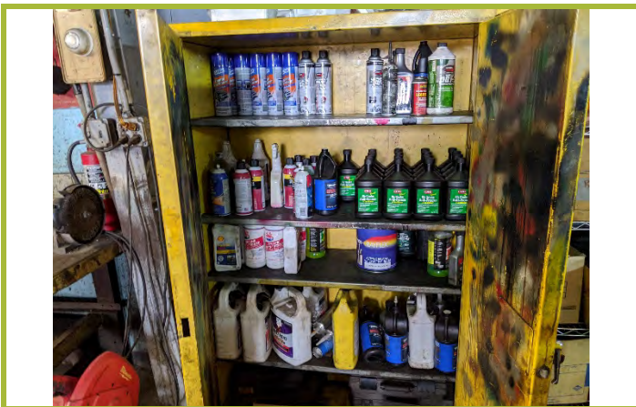
Photo #5: Flammable storage cabinet in Maintenance Garage.
