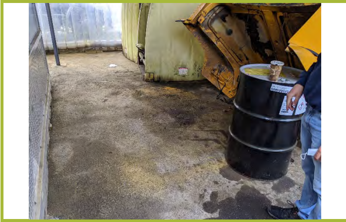
Photo #13: Staining and drums observed in storage sheds.
