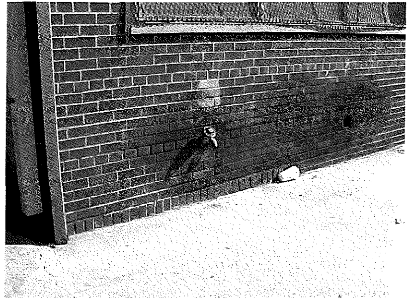
Picture #14: View of the fill cap and vent pipe associated with a former trichloroethylene UST which was closed in-place on-site.
