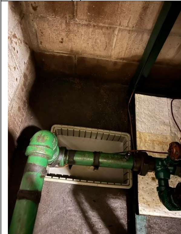
Spill Tray in Subject Property Elevator Equipment Room
