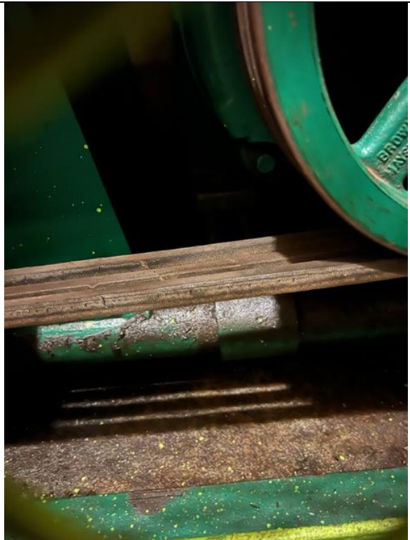
Subject Property Elevator Equipment Room
