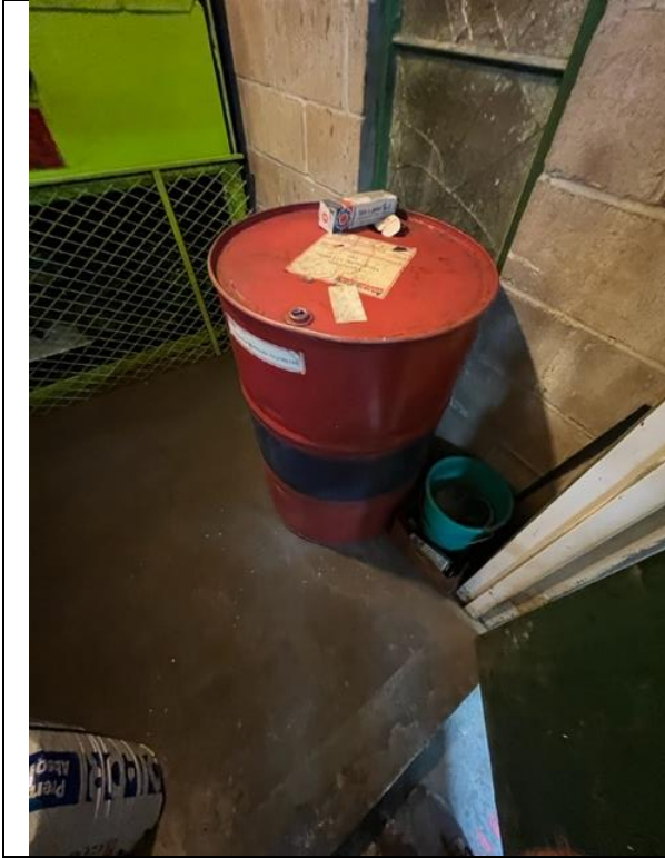
Drum of Hydraulic Oil In Subject Property Elevator Equipment Room
