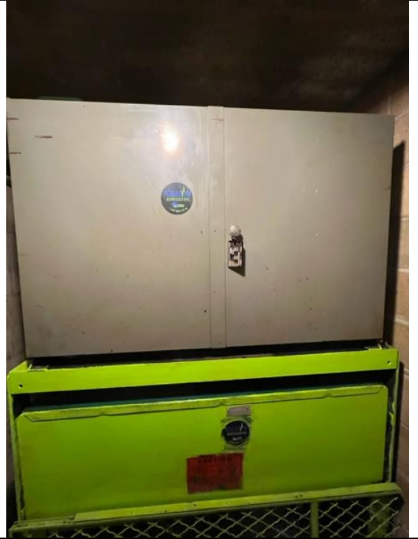
Subject Property Elevator Equipment Room
