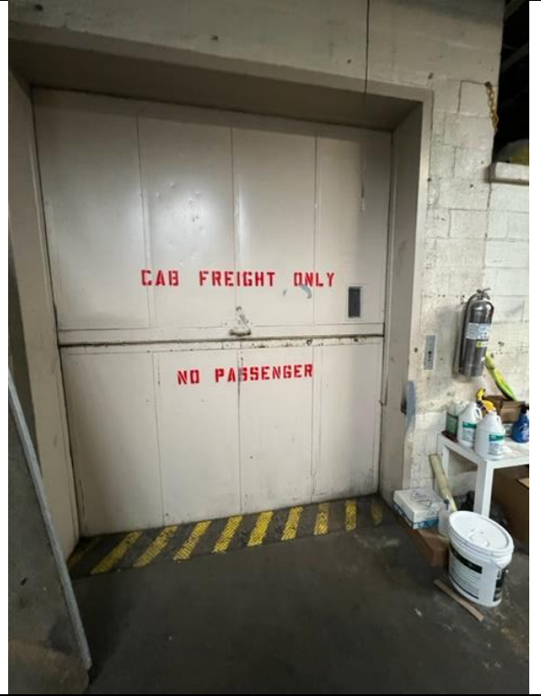
Subject Property Hydraulic Elevator
