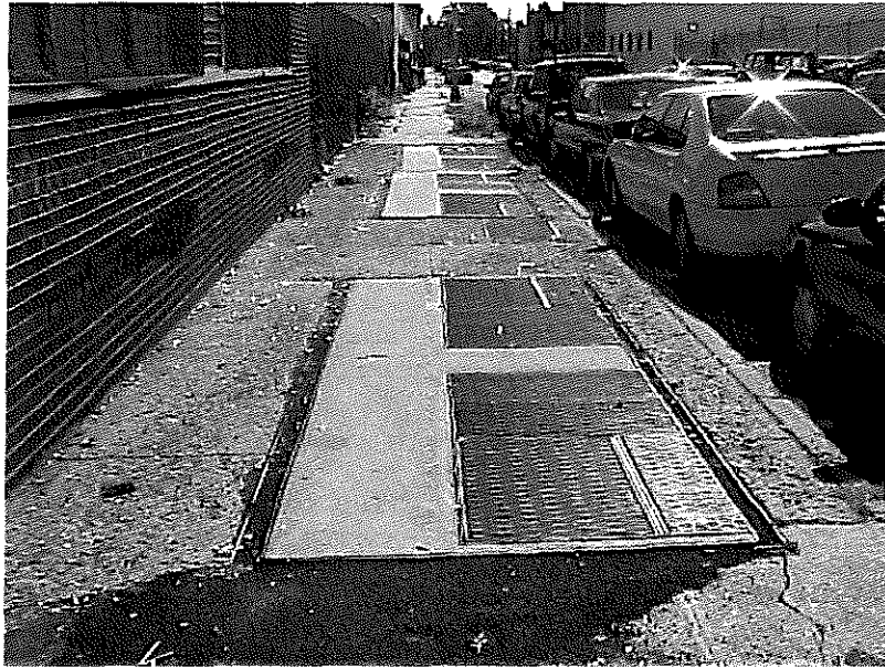
Picture #21: View of the vaulted transformers located on the sidewalk in front of the subject property.
