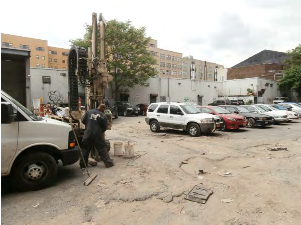
Photo 6 – Location of soil boring B-4 in the southern portion of parking lot.
