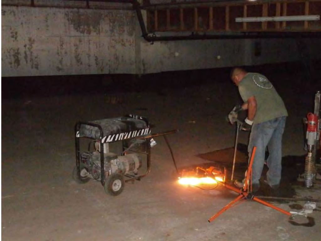
Photo 11 – Zebra hand drilling B-8 in southern section of garage near location of former UST.
