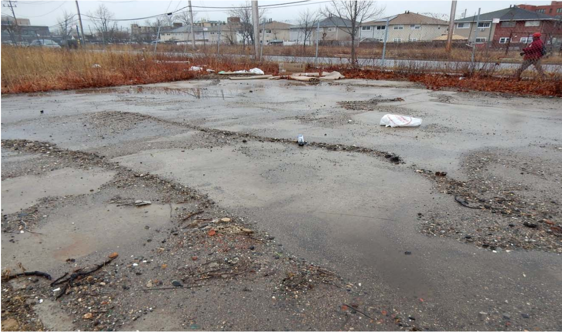
View of the concrete slab associated with the former structure at the northwestern corner of the site, looking southwest.
