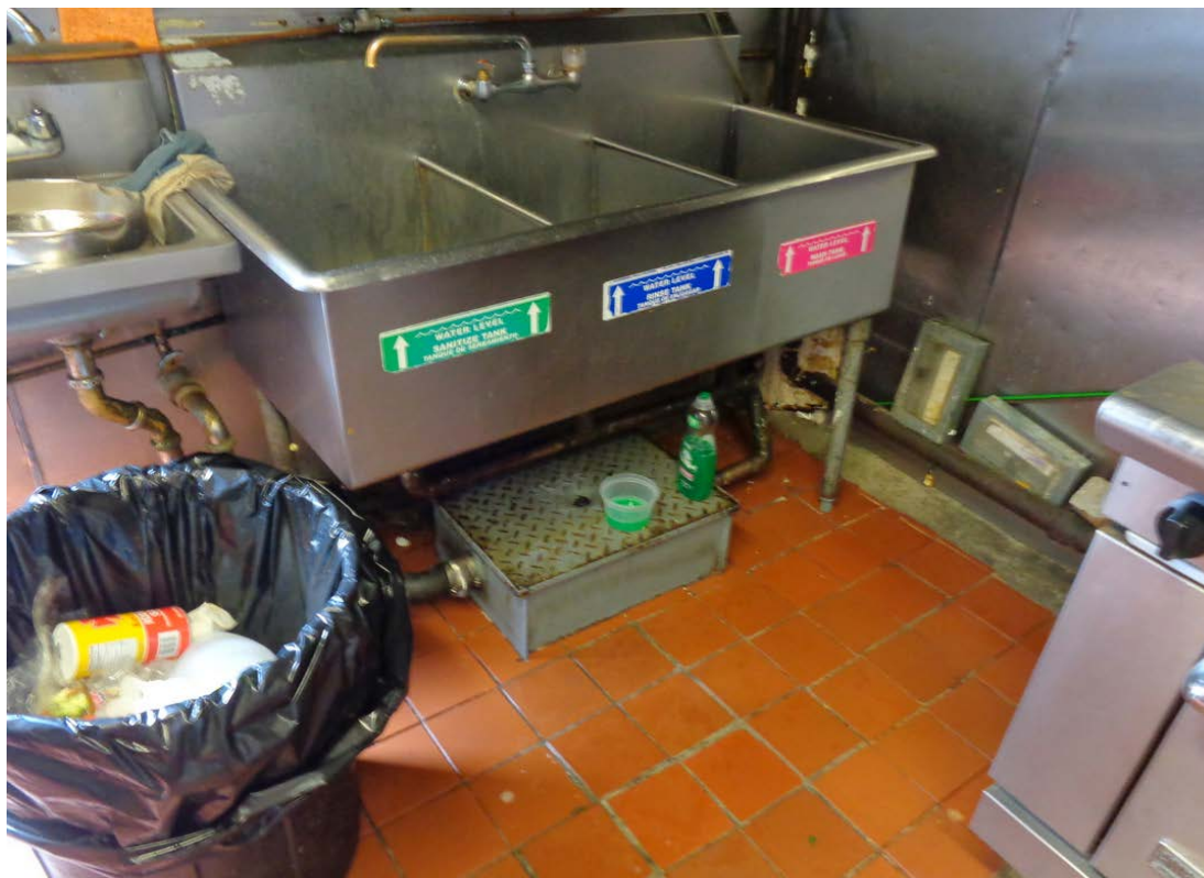
Figure 4: The grocery/supermarket includes three grease traps to collect waste cooking grease.
