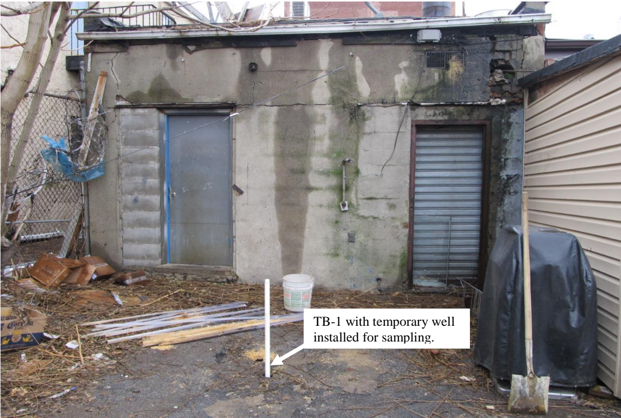
Figure 3: Completed TB-1 temporary monitoring well with installed 2-inch diameter, schedule 40 PVC well casing with 5.0-feet of 0.01" slotted screen.
