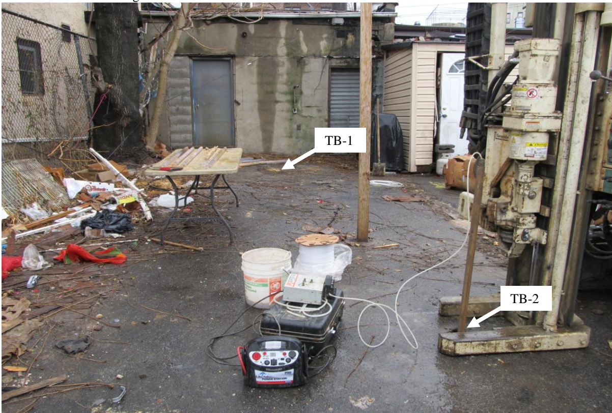
Figure 6: Another view of TB-2 relative to the rear of 1322 Central Avenue and TB-1. This view is looking southeast. Boring TB-2 collapsed after the soil cores were removed and before a temporary well could be installed. The boring was redrilled using an SP-15 hydropunch to collect the groundwater sample. Elevated tetrachloroethylene was detected in both TB-1 and TB-2.
