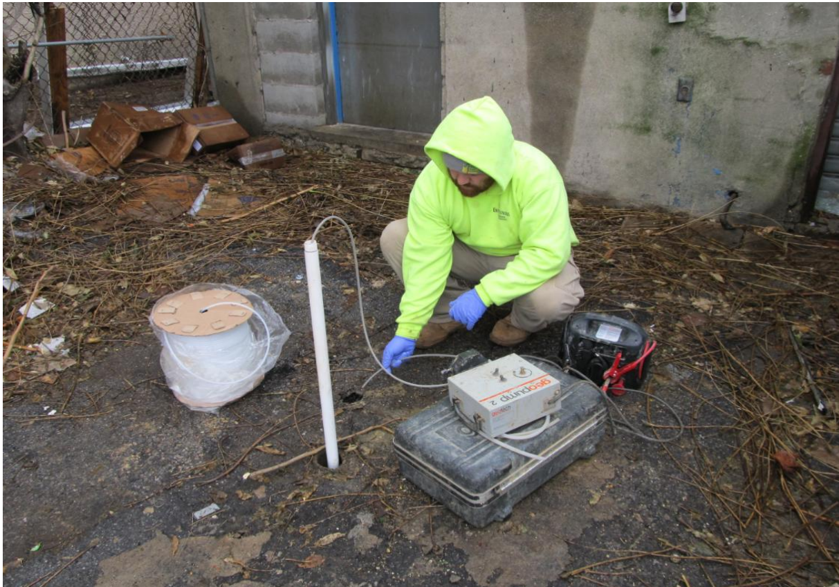
Figure 4: Development of the temporary well at TB-1 using a Geopump 2 peristaltic pump and new polybutylene and Teflon tubing. Abundant groundwater are produced at all test locations by an unconfined aquifer at ~21.0-feet below ground surface (bgs).
