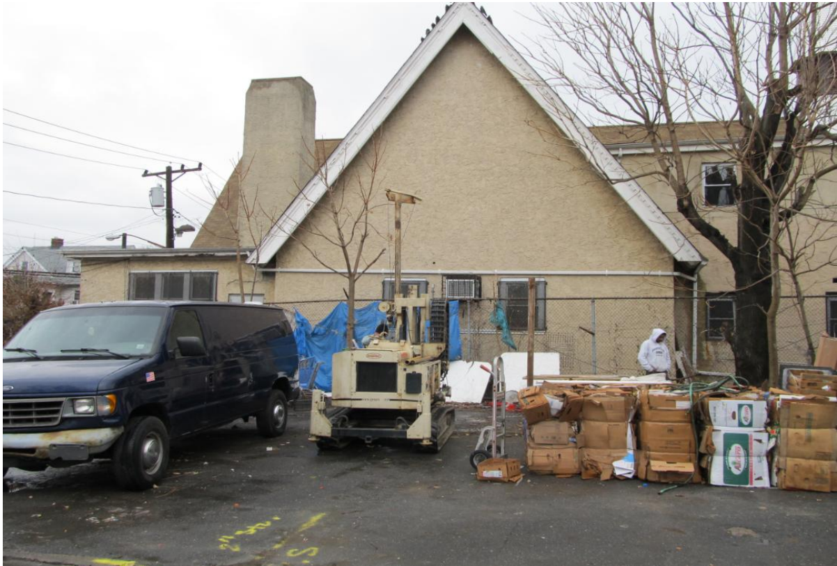
Figure 5: Completion of TB-2 farther southwest from the rear of 1322 Central Avenue. This view is looking northeast. The adjacent Church of God is visible in the background.
