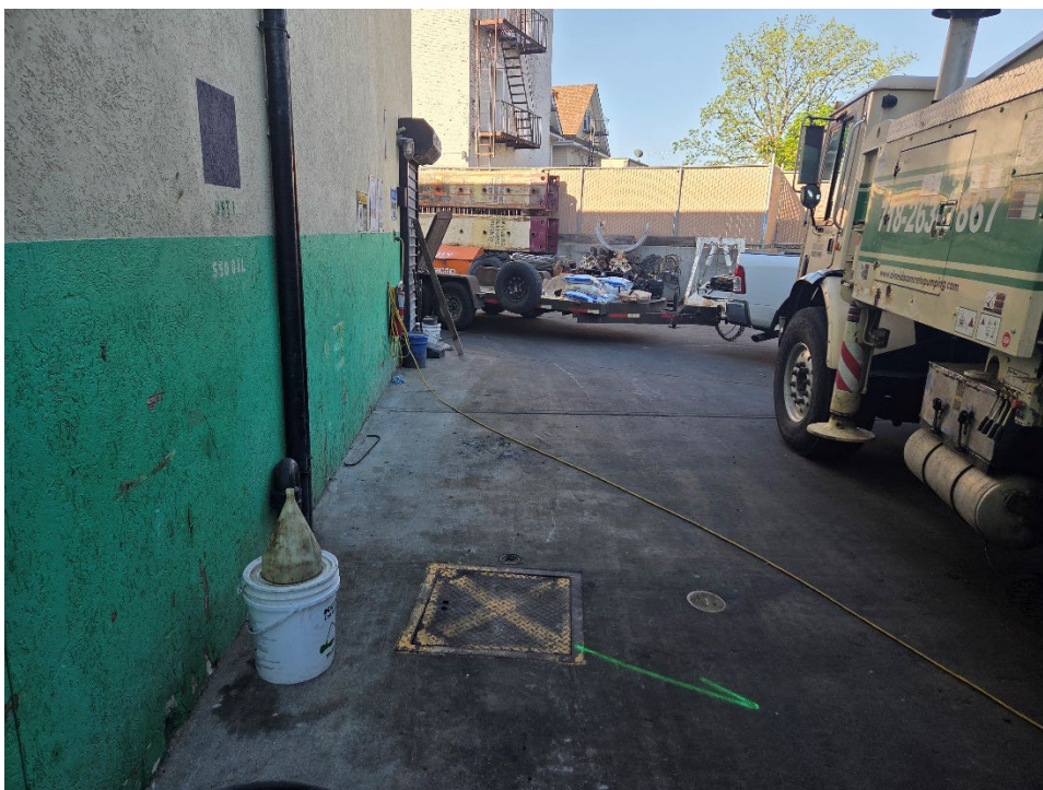
Photo 6. Fill port and access hatch above a known UST detected outside of the building.
