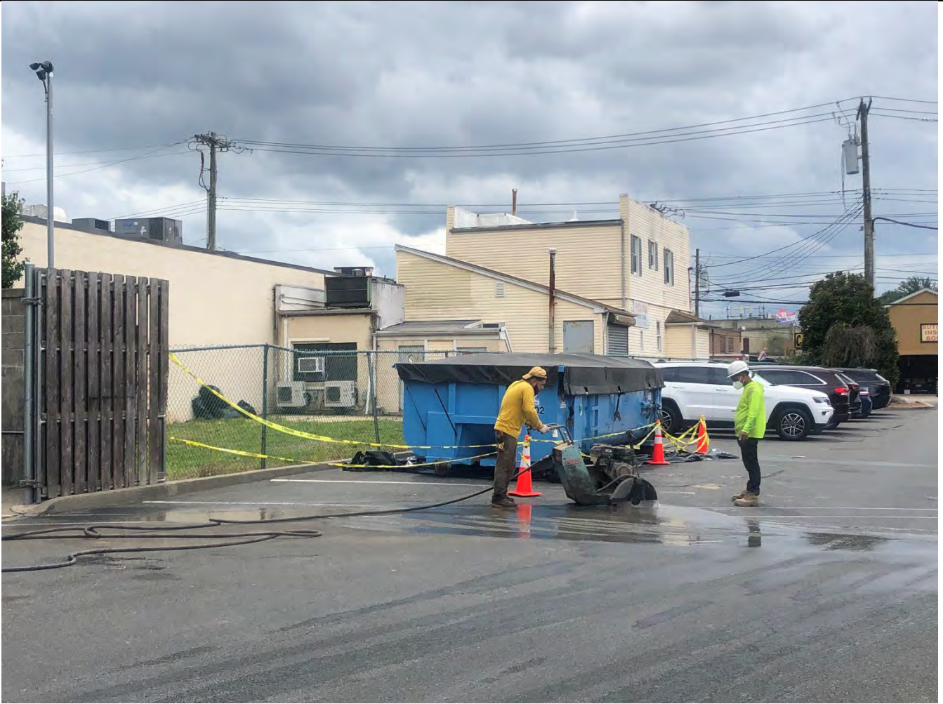
Photo 3: Looking south. View of Carmine wet saw cutting second trench in preparation for excavation the following day.
