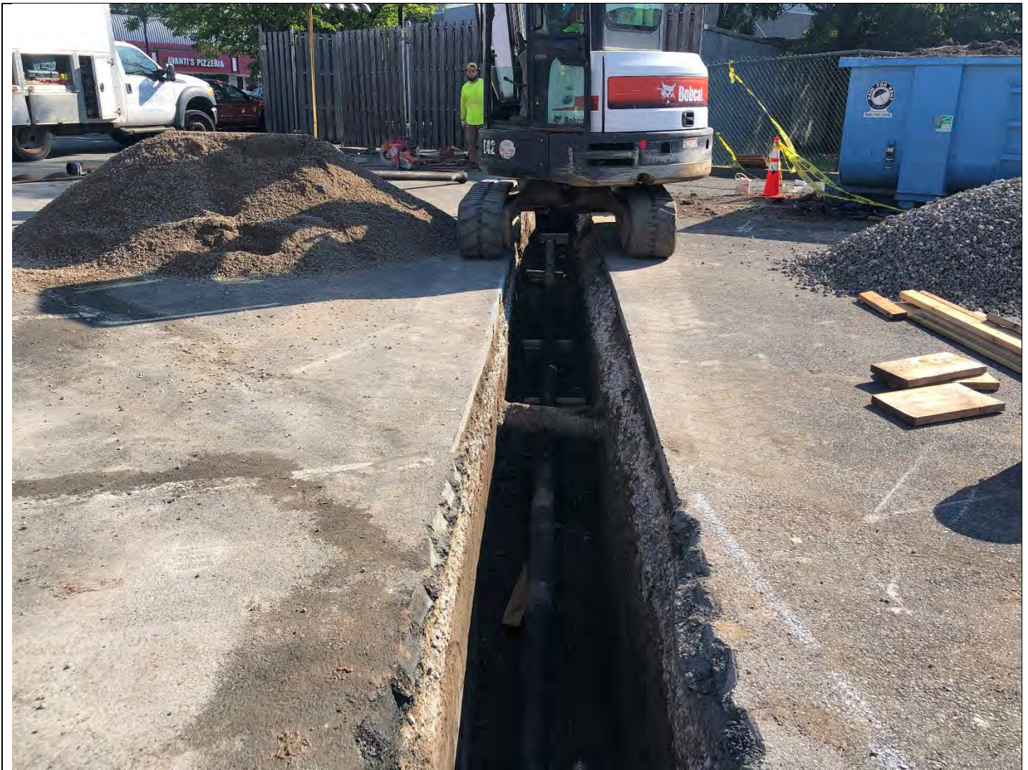
Photo 2: Looking east. View of new sewer line piping placed inside of trench.
