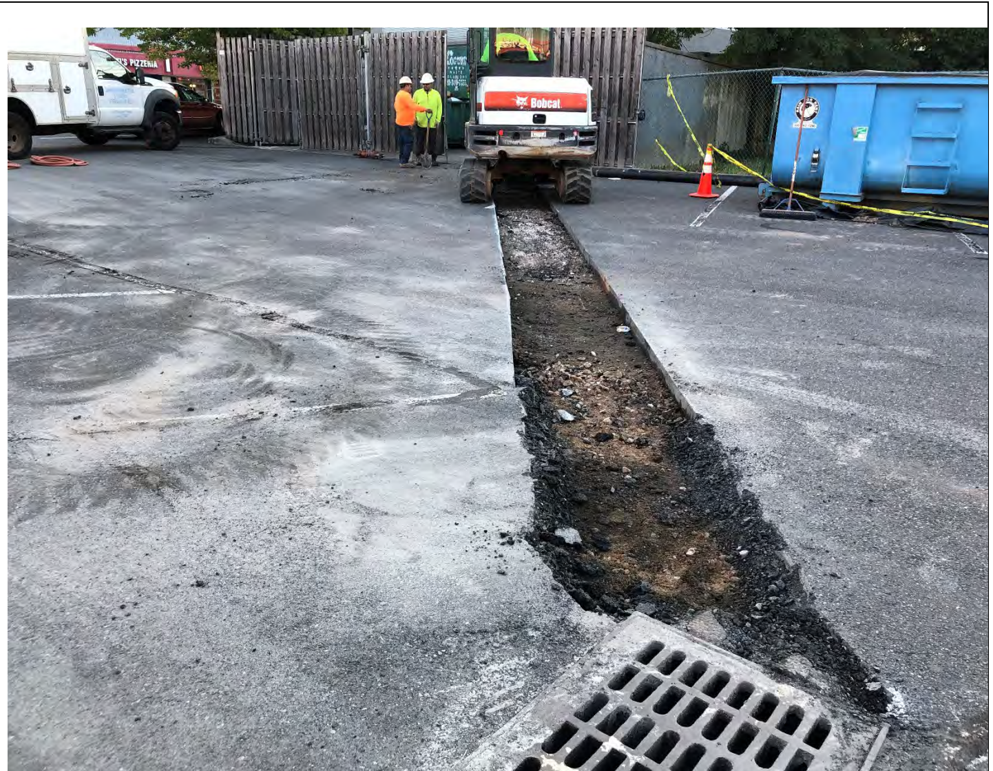
Photo 1: Looking east. View of beginning of excavation for second sewer line replacement.
