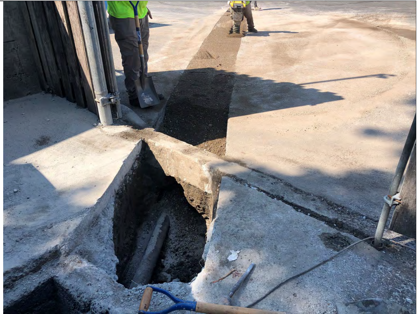
Photo 3: Looking west. View of new sewer piping with backfilled material and workers compacting material.
