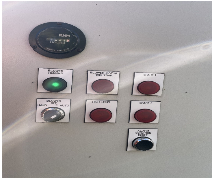
Photograph 7: View of SSDS runtime meter and running light.
