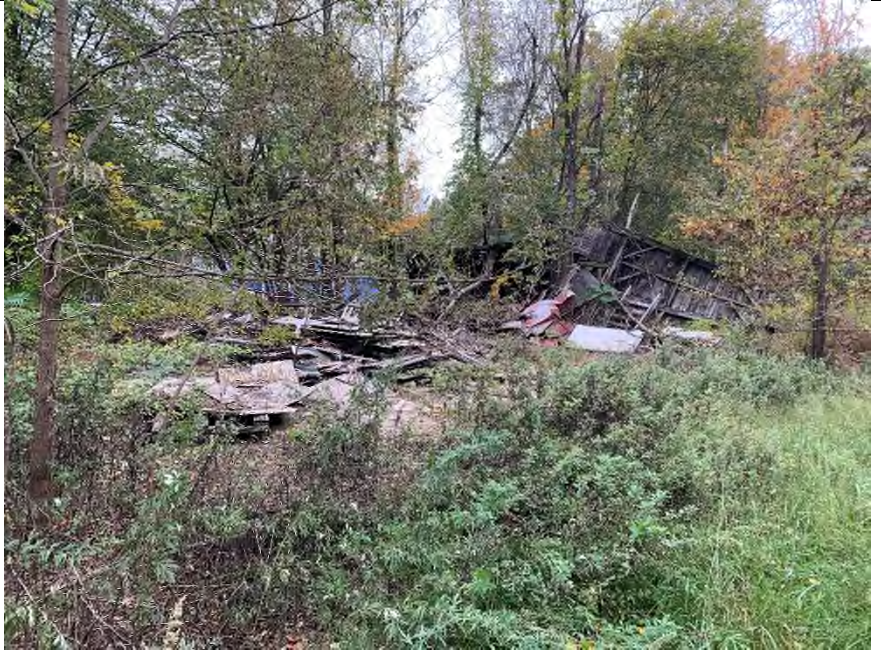
Photo 1 – Auto Garage East (Collapsed).
