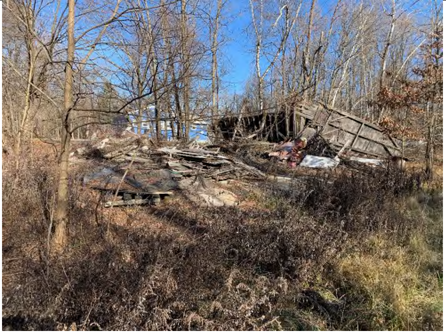
Photo 1 – Auto Garage East (Collapsed).
