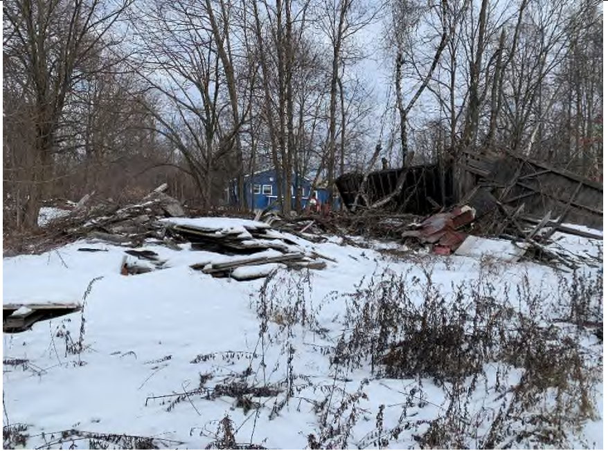
Photo 1 – Auto Garage East (Collapsed).
