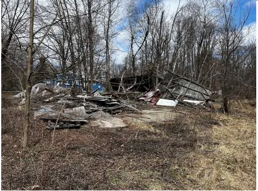
Photo 1 – Auto Garage East (Collapsed).
