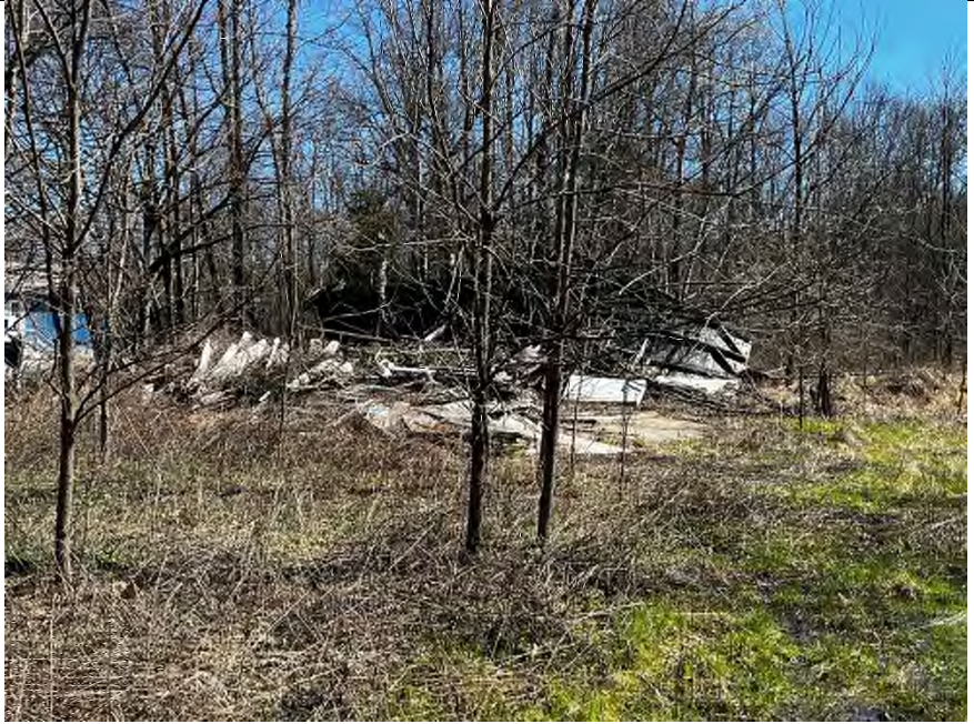
Photo 1 – Auto Garage East (Collapsed).
