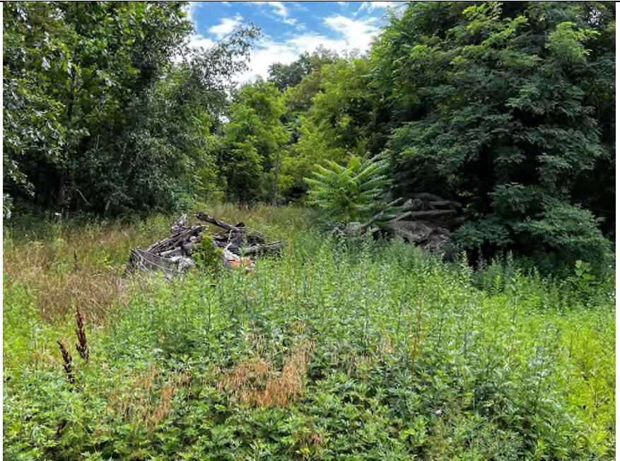
Photo 1 – Auto Garage East (Collapsed).
