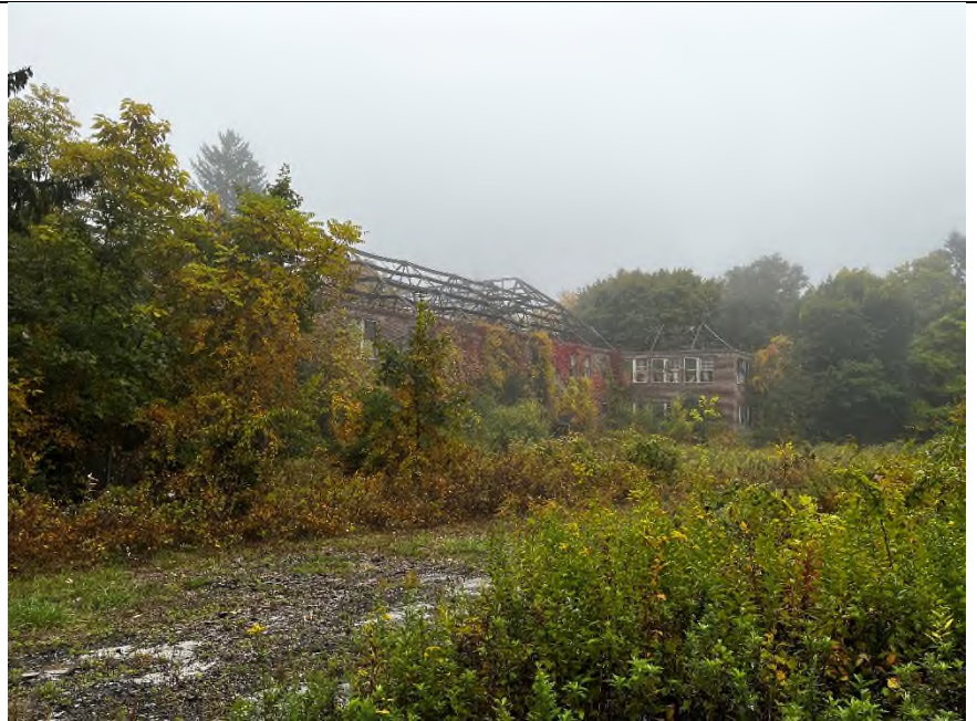
Photo 16 – Brookside structure, severe deterioration of roof.
