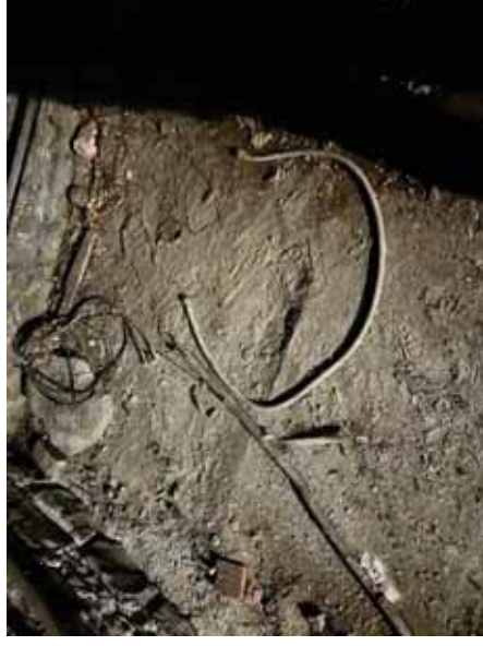
8. Discarded fuel line, basement, Lot C
