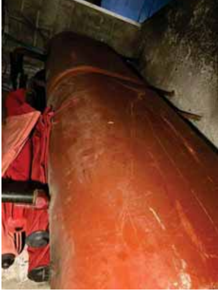
5. Two disconnected, empty, manifolded 275-gallon fuel oil tanks, eastern side of basement, Lot A
