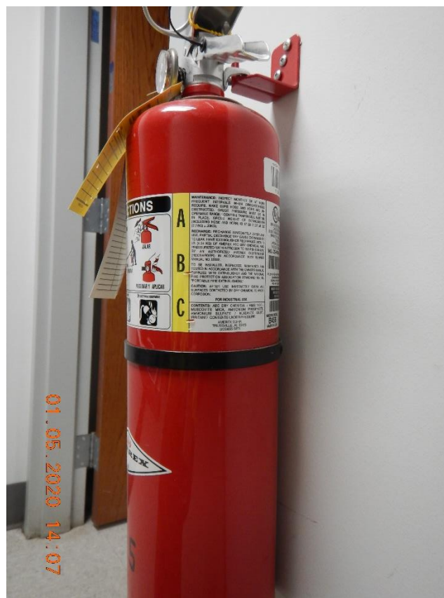
Photo 22: Office Fire Extinguisher
