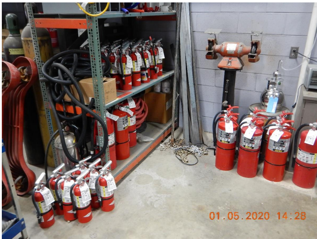
Photo 12: ABC Fire Extinguishers, Air cylinders
