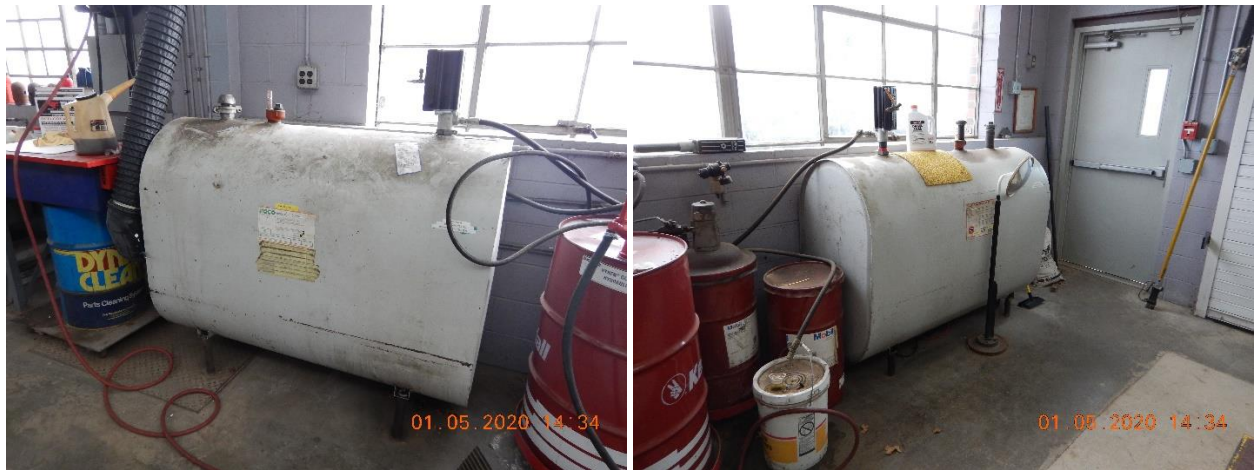
Photo 7: 275-Gal Motor Oil Tanks
