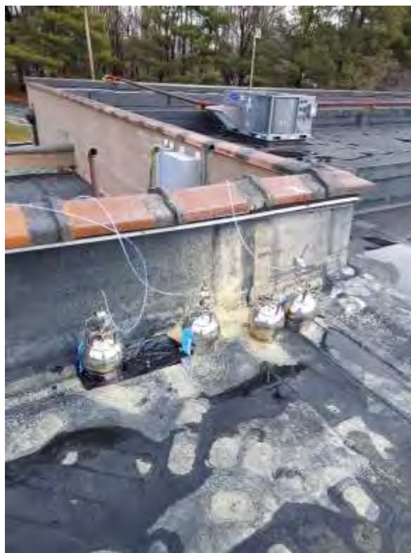
Photo 64: Blower 1, Blower 2, Blower 3, Blower 3D
