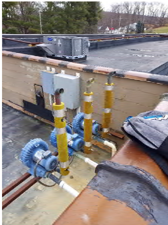
Photo 4: Upgraded blowers now equipped with insulation, temperature gauges, and effluent sample ports.
