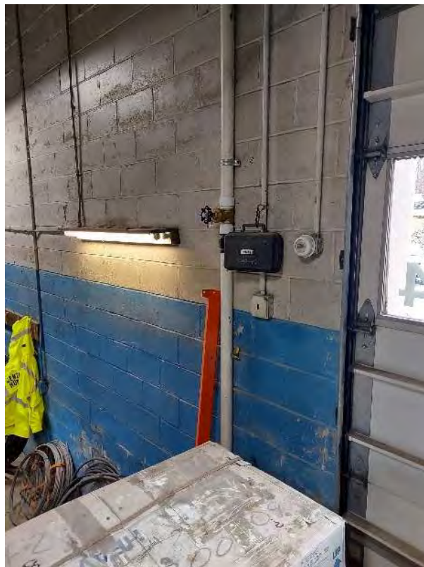
Photo 45: Extraction Well 3 Riser
