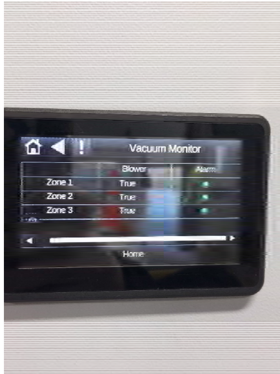
Photo 5: LCD Display on Pressure Switch Housing
