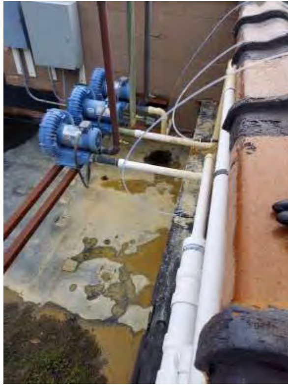
Photo 65: Blower Sampling Connection Locations
