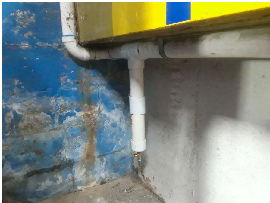
Photo 2: Example of Drain Port - EW-3
