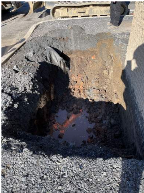
11 - Water encountered in excavation 03.21.2022
