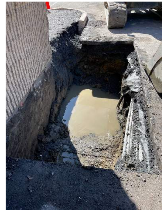
12 - Water encountered in excavation (2) 03.21.2022
