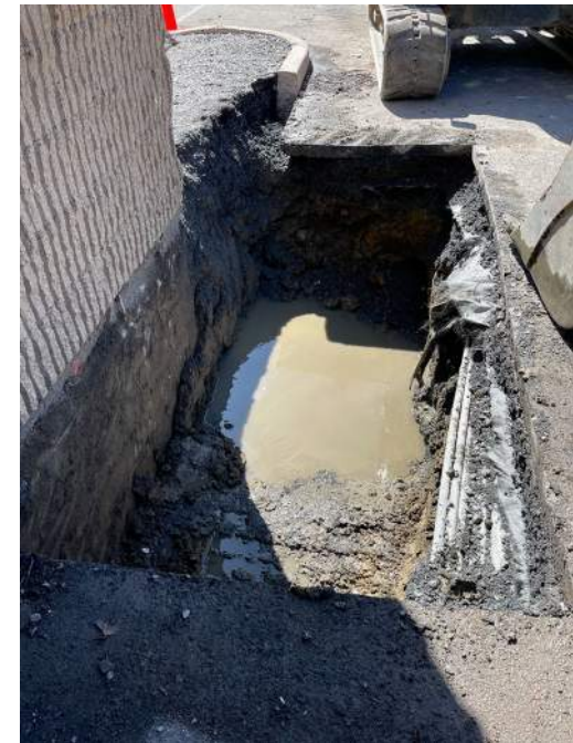
12 - Water encountered in excavation (2) 03.21.2022
