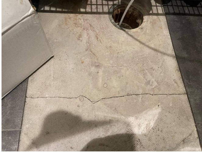
(Before photo) Crack identified in the concrete floor slab in Area 2.
