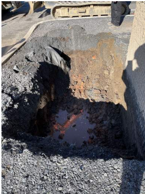
11 - Water encountered in excavation 03.21.2022
