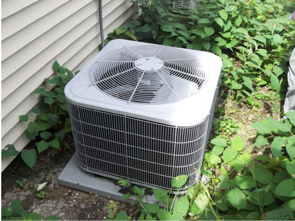
View of additional air-conditioner condenser unit for office area.
