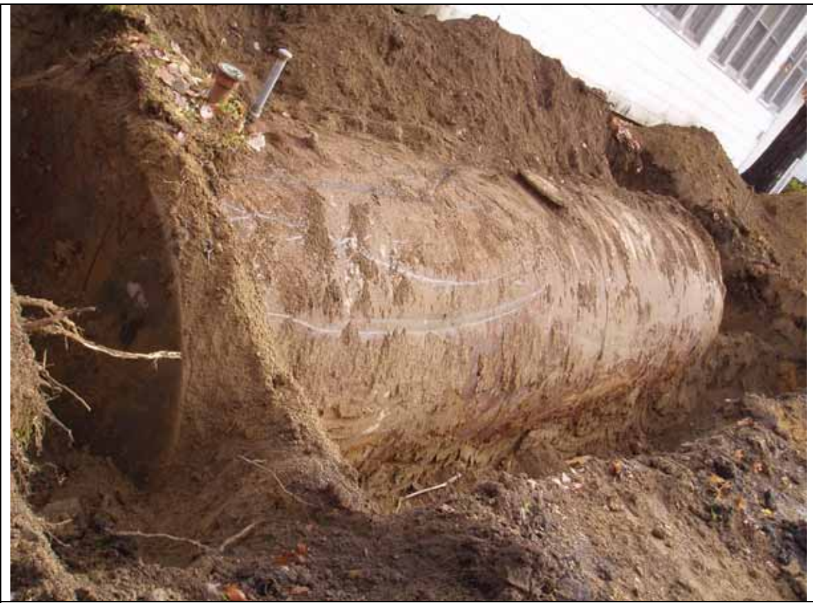
Mobile Media, 24 Center Street, Pine Bush, New York Removal Of 10,000 gal. Fuel Oil UST In Progress
