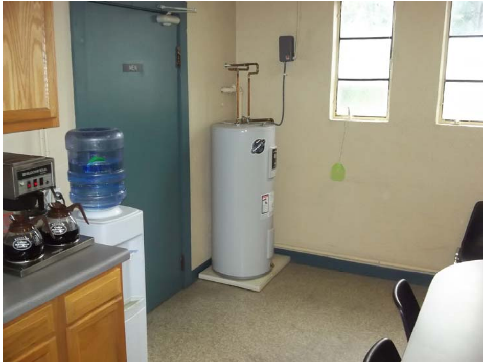
View of hot water heater in break room.
