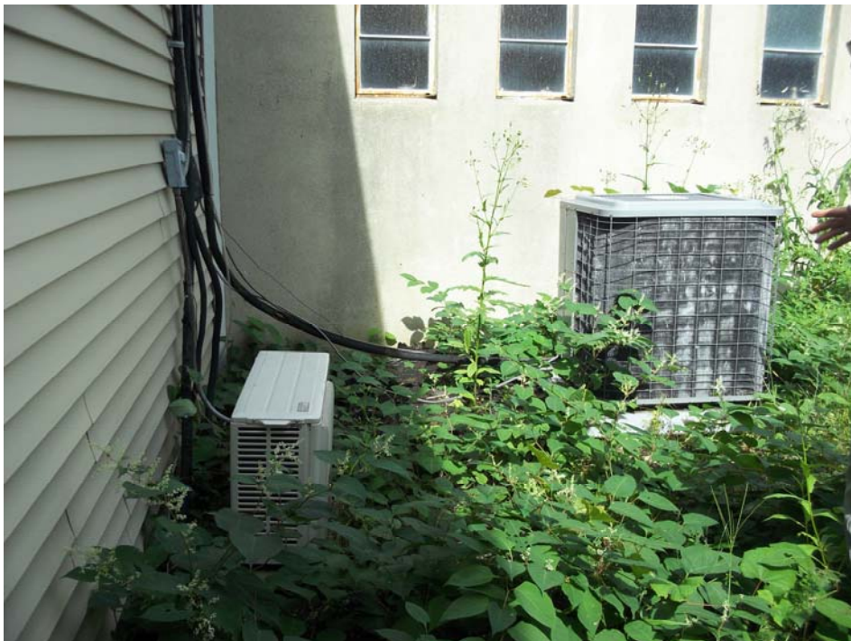
View of two (2) air-conditioner condenser units for office area.
