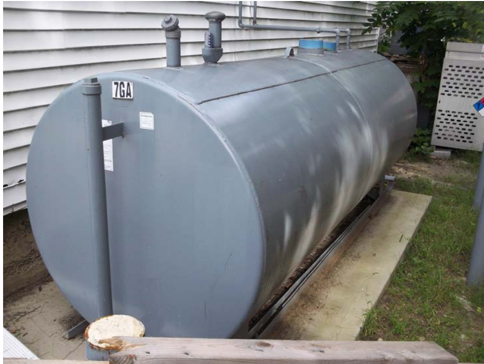
View of one (1) 1,000-gallon #2 fuel oil AST to supply boiler for shop area.
