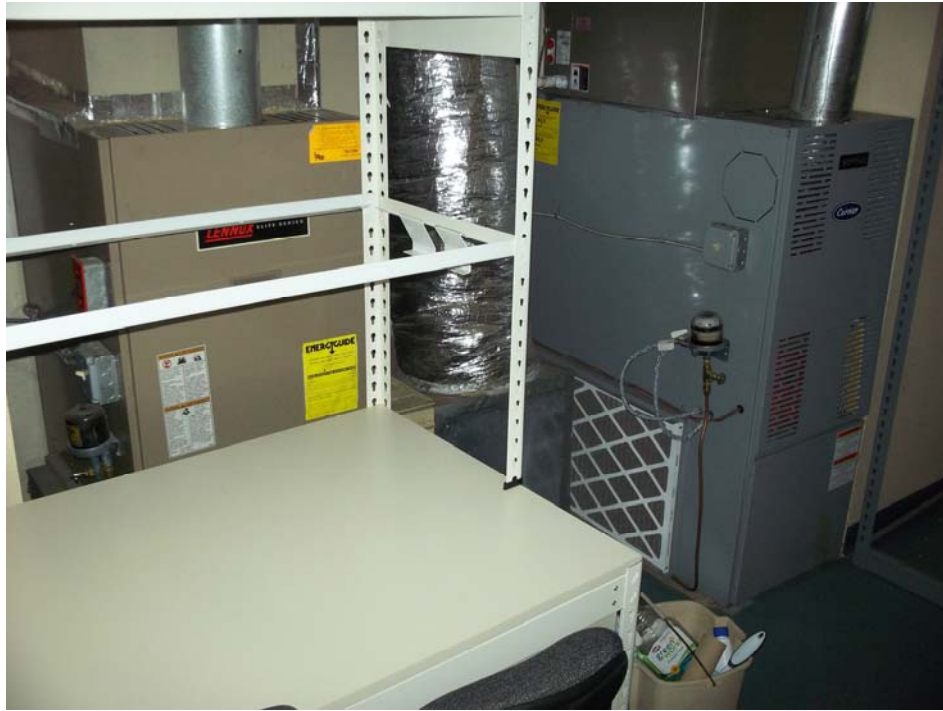
View of two (2) furnaces in hallway to supply heat to office areas.
