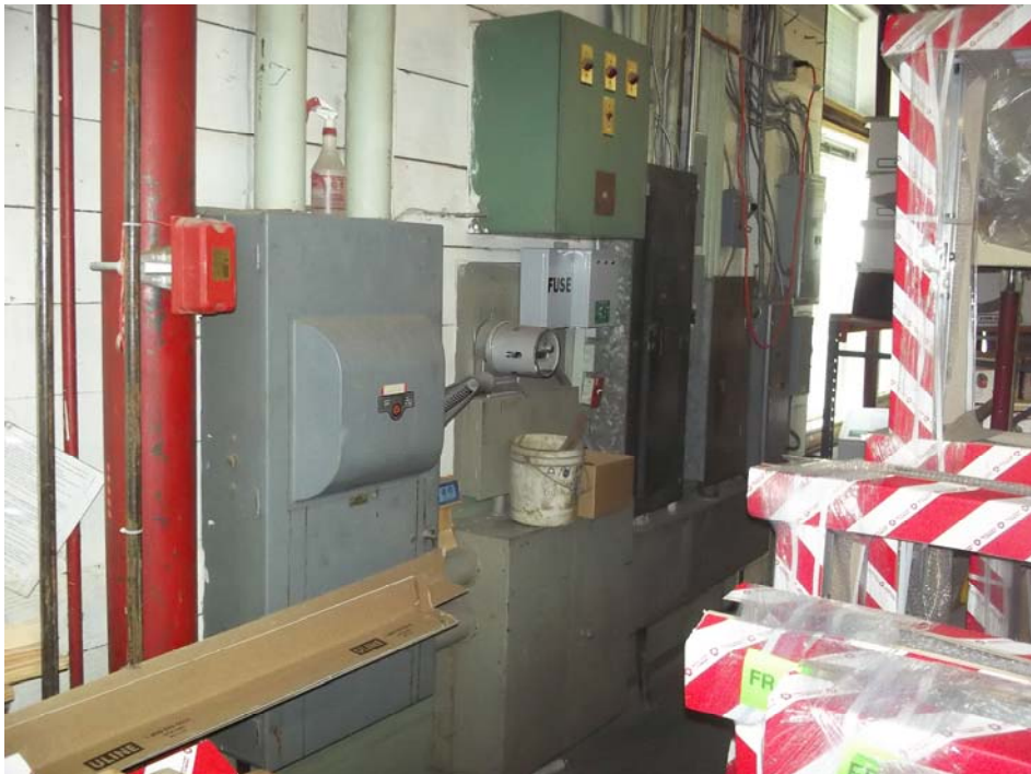
View of electric meter in shop area of subject building.
