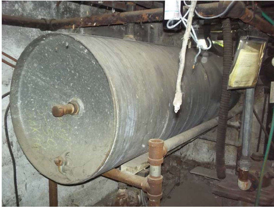
View of inactive steam tank in boiler room, reportedly associated with former site operations.
