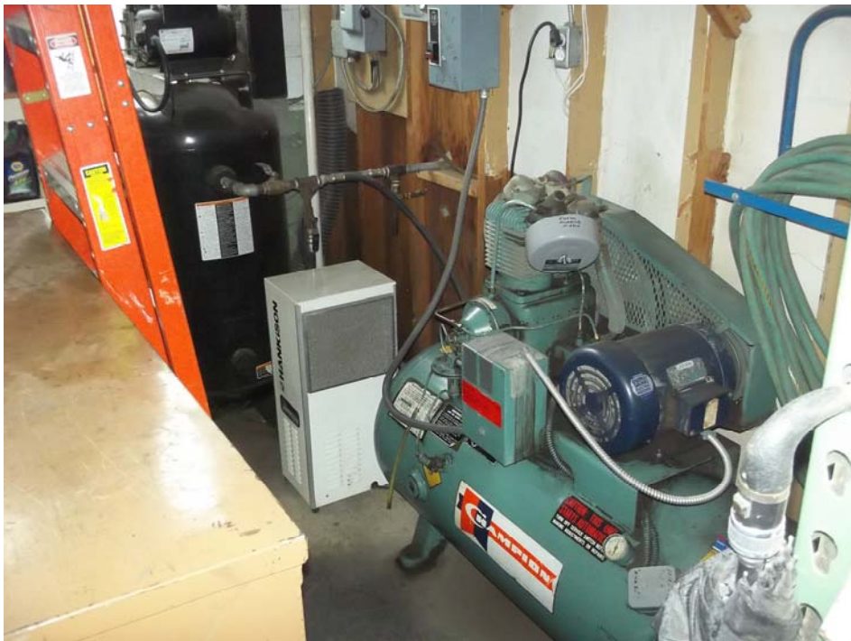
View of air compressors in shop area.
