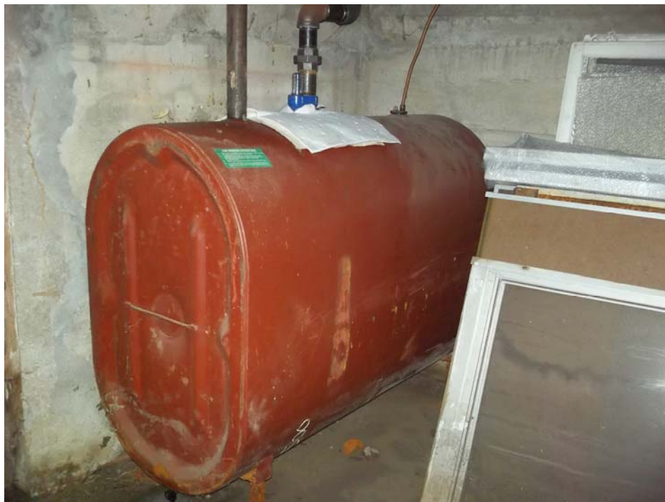
View of 275-gallon #2 fuel oil AST located in basement area to supply two (2) furnaces utilized to heat the office area.
