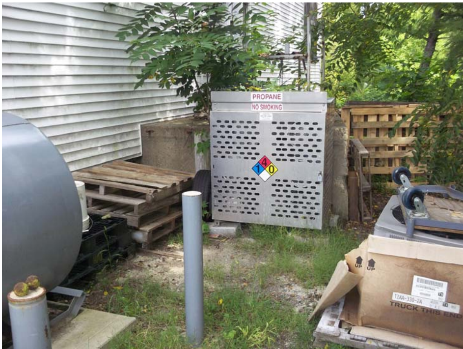
View of forklift propane tank storage to east of subject building.
