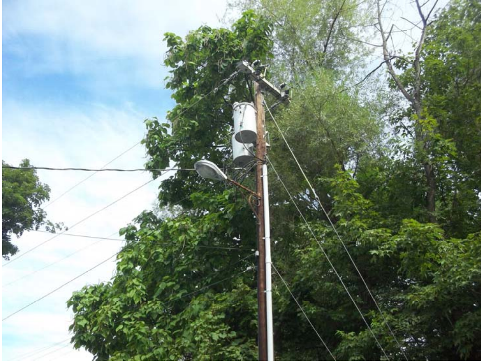
View of two (2) pole-mounted transformers near southeast corner of subject property.
