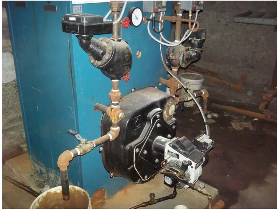
View of boiler located beneath shop area, which supplies heat to shop area.
