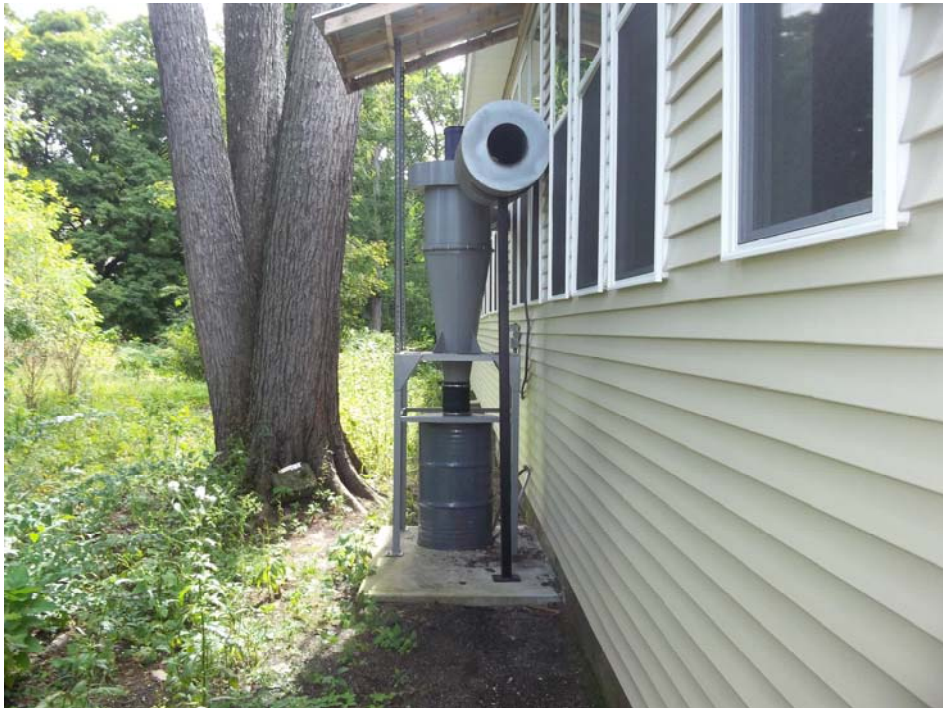
View of metal shavings collection canister/drum on north side of subject building.
