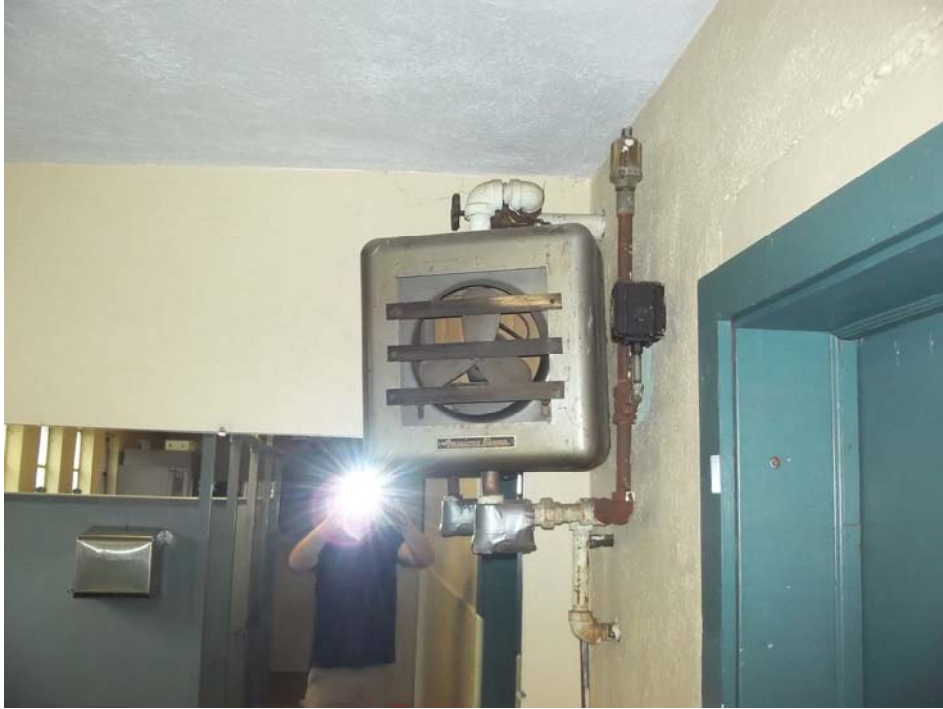
View of steam heater in men's restroom.
