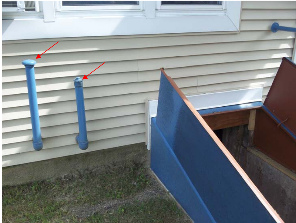
View of access to basement area, beneath office area. Note the locations of the vent and fill pipes associated with the 275-gallon AST in basement area.
