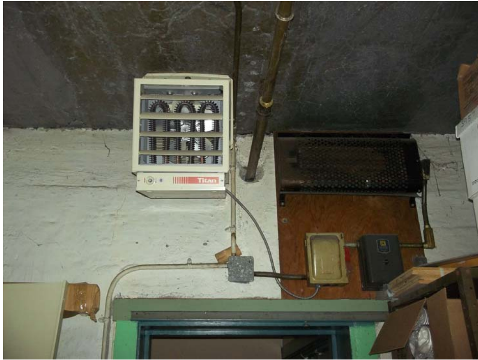
View of electric heater in storage room.
