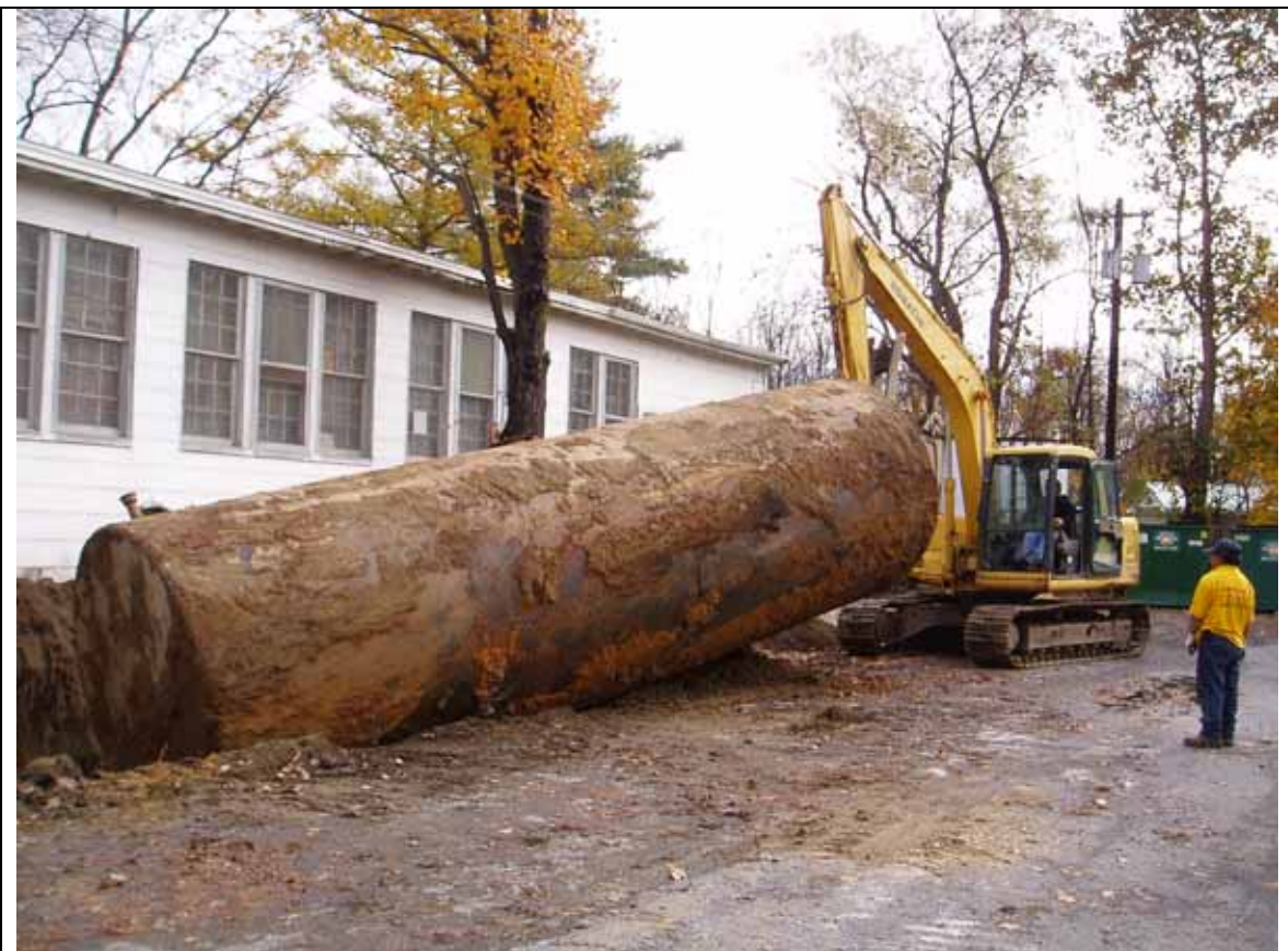
Mobile Media, 24 Center Street, Pine Bush, New York Removal Of 10,000 gal. Fuel Oil UST In Progress
