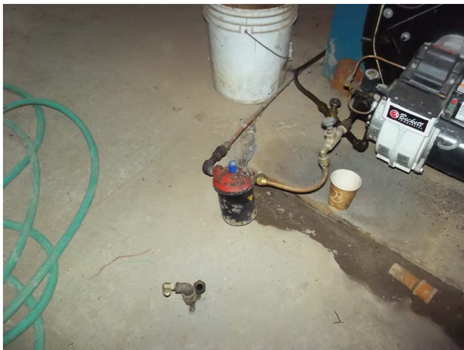
View of fuel oil lines protruding from concrete floor in boiler room, reportedly associated with the former 10,000-gallon UST.
