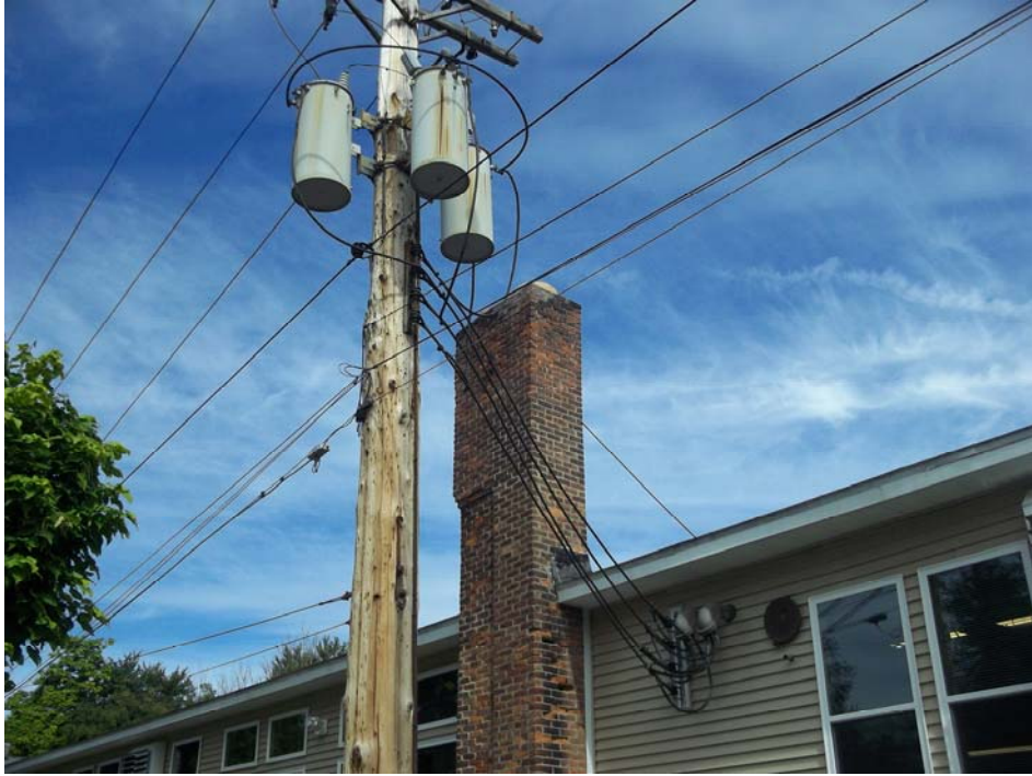
View of three (3) pole-mounted transformers to south of subject building and electric entering subject building.
