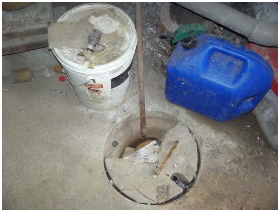
View of reportedly inactive sump pit in boiler room.
