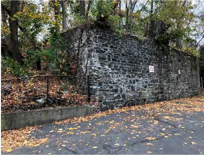
5. Foundation remains, northeastern corner; as viewed from the eastern adjoining property, facing west
