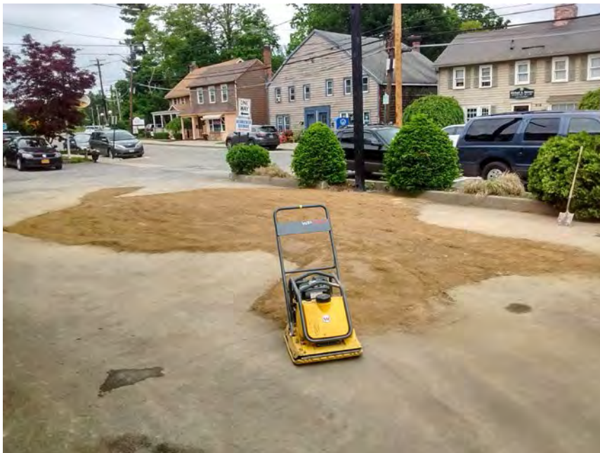
18. Looking northwest across excavation area after being backfilled with clean fill and compacted
