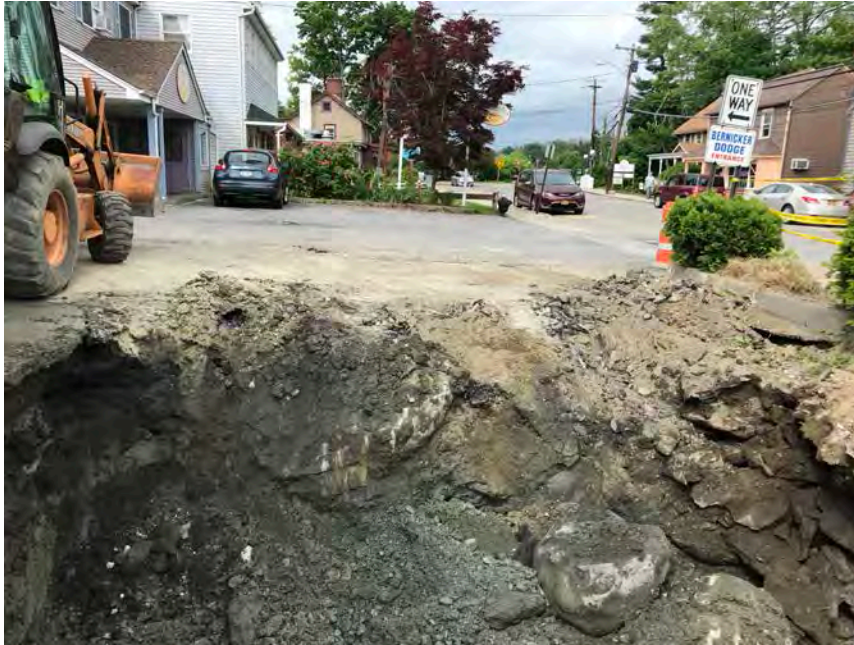
11. Western edge of excavation area; further work was impeded by the presence of large boulders and subsurface utility lines
