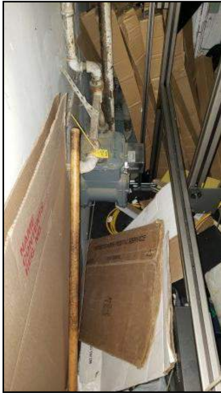
View of the natural gas meter located in adjacent to the entrance of "Generations Thrift Emporium".
