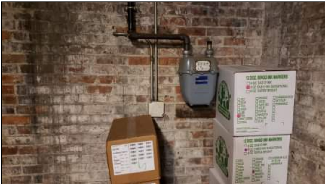
View of the disconnected natural gas meter located in the decommissioned boiler room.
