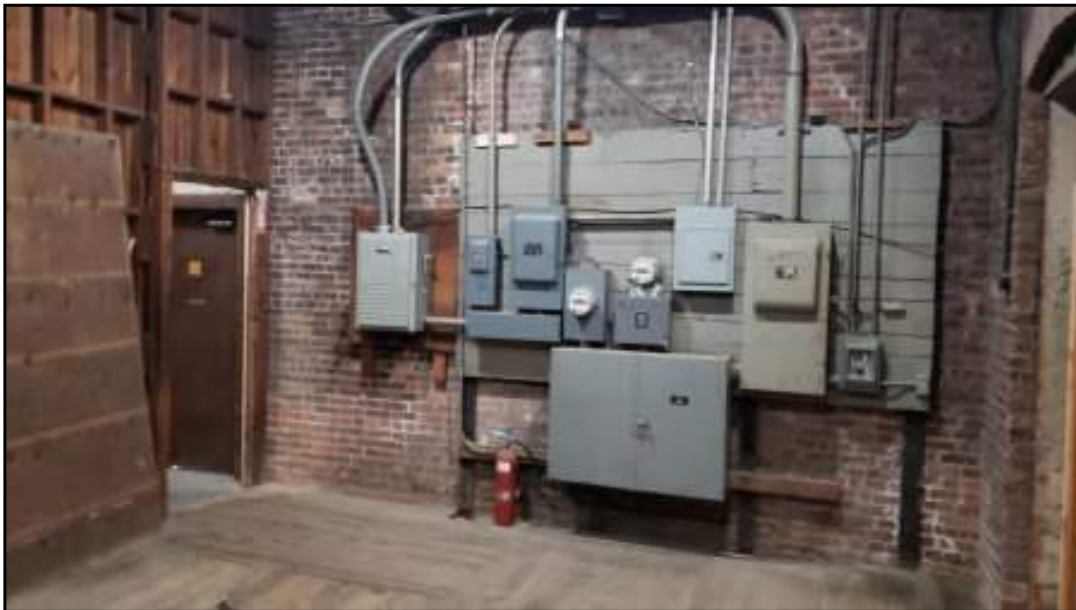
View of electric utilities located in the southwest corner of the first floor.
