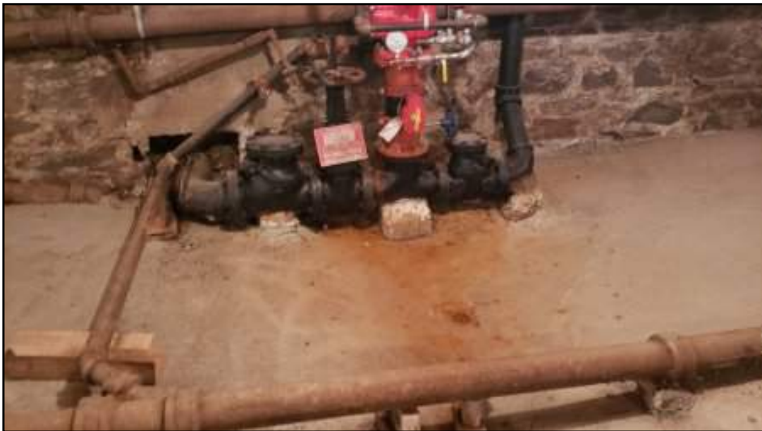
View of the floor drain and sprinkler system located in the northern section of the basement in the on-site building.
