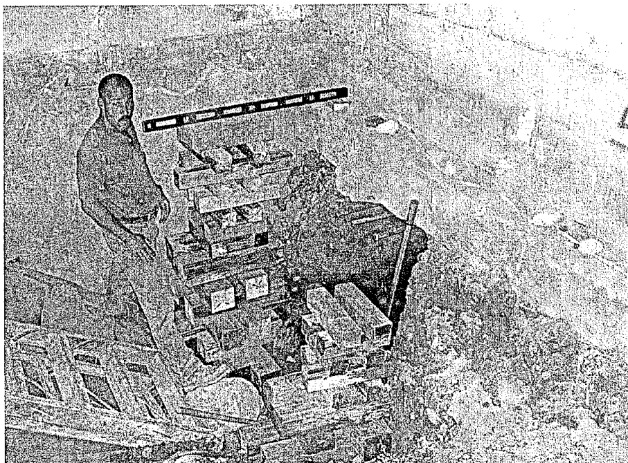
Photograph #10 - Spiriks Contracting employee use a level while building the wooden cribbing which was used to support the steel pins during the underpinning of the northern wall of the Chromium Room.
