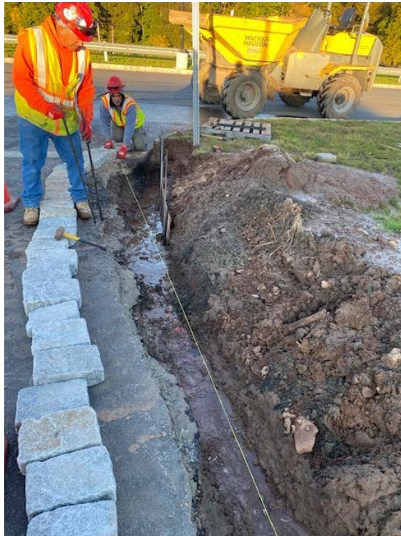
Photo 1: Placing forms in ground at Building G area in preparation for concrete pour.
