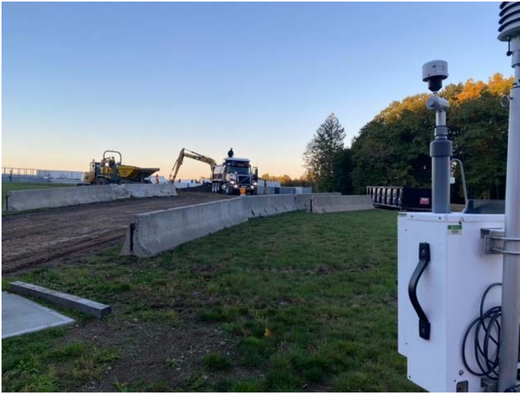
Photo 1: Backfill one of two access ramps to northern trailer area and place demarcation.
