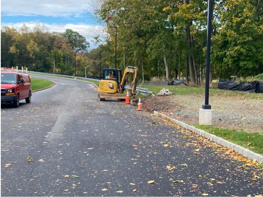
Photo 1: Clearing out curb excavations filled with water from nor'easter on previous day.
