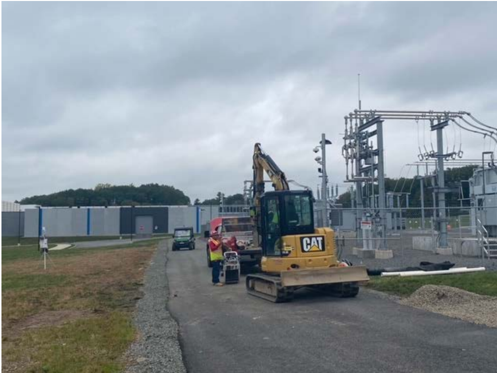
Photo 2: Work stopped due to equipment failure.
