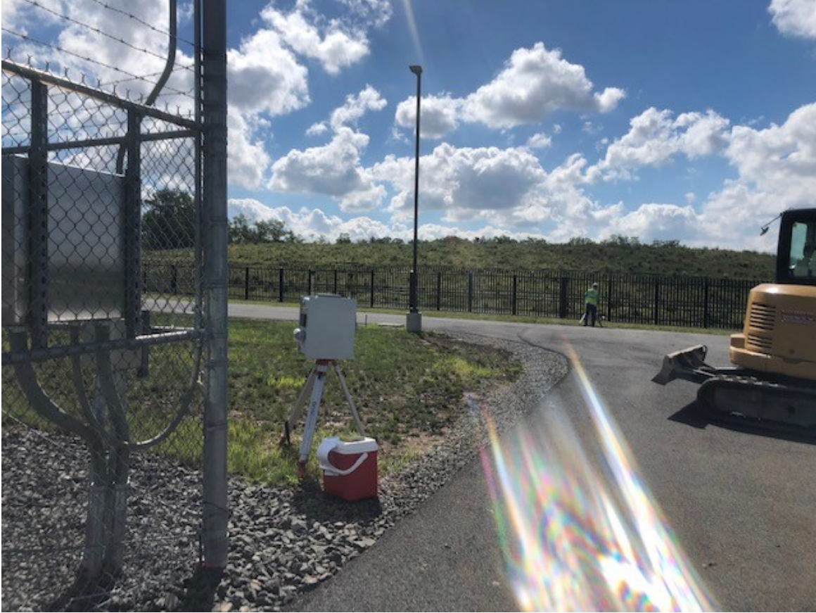
Photo 1: CAMP setup at substation.
