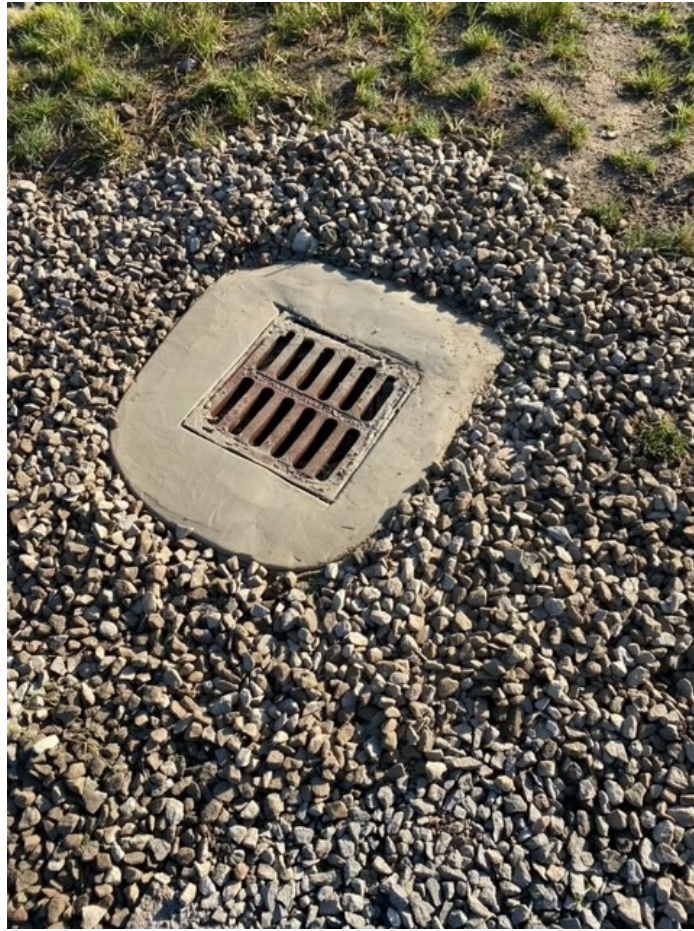
Photo 1: Cement over drainage pipe at substation and refit drainage pipe in soil.
