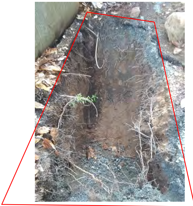
10. TP-10 (275-gallon AST at left)
