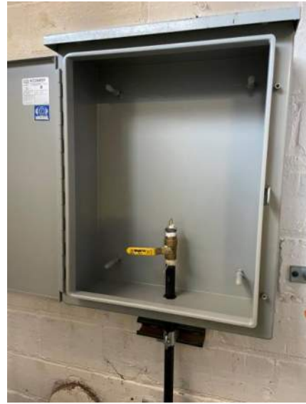
Nonfunctioning sampling port
