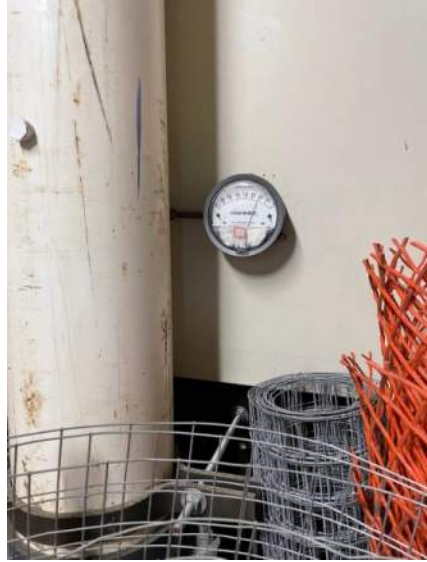
Gauge requiring replacement
