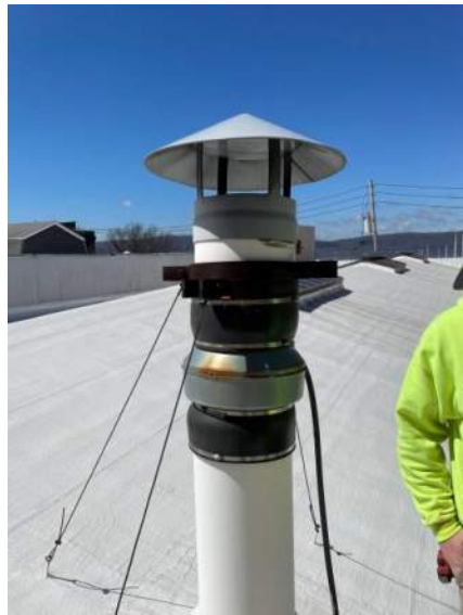
Roof mounted inline fan
