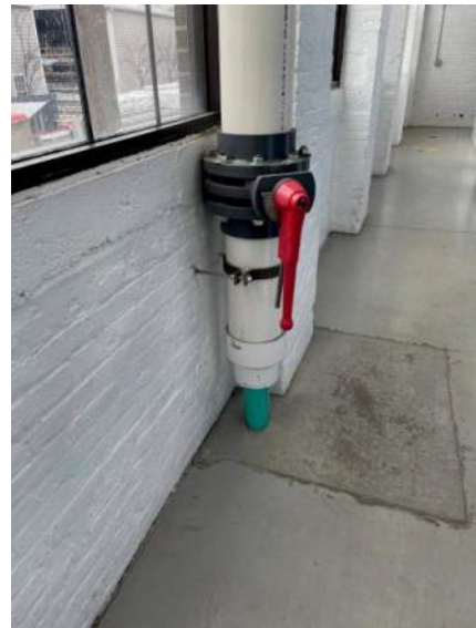
Conveyance piping and valve
