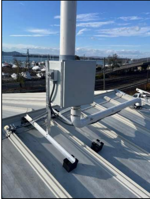
System Blower and Exhaust
