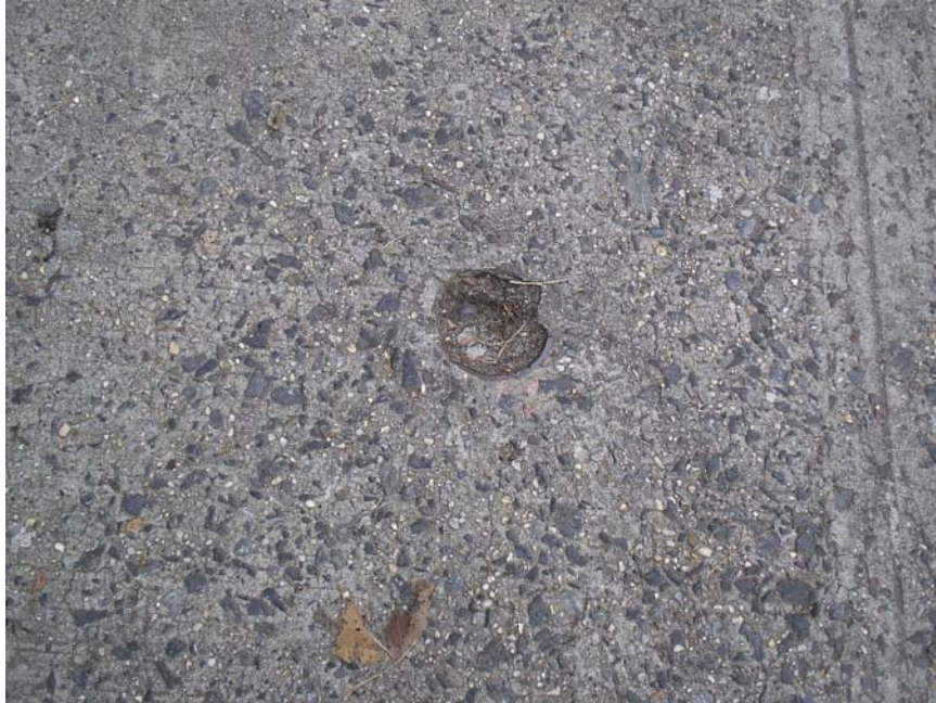
Photograph 7: Inactive Fill Pipe in the Sidewalk
