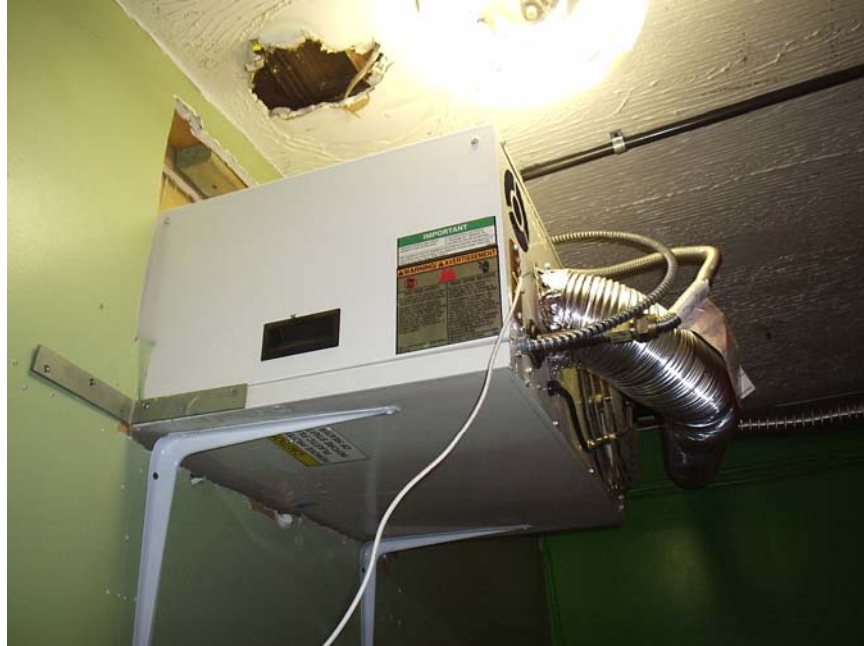
Photograph 5: Overhead Natural Gas Fired Heating Equipment
