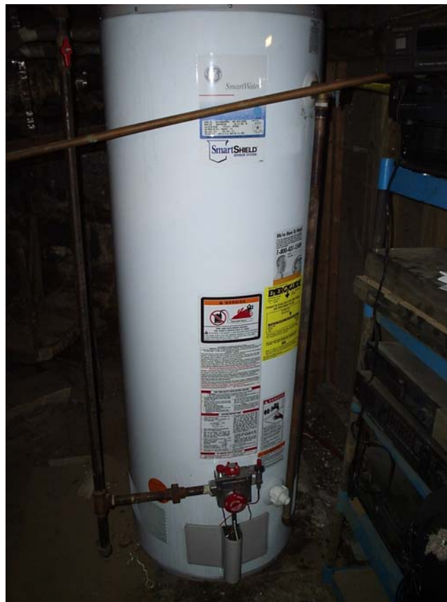
Photograph 6: Natural Gas Fired Hot Water Heating Equipment
