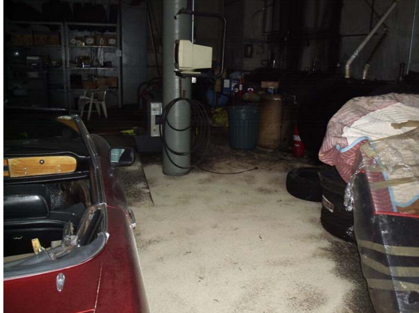
Photograph 7: Tank Room Floor and Oil Staining
