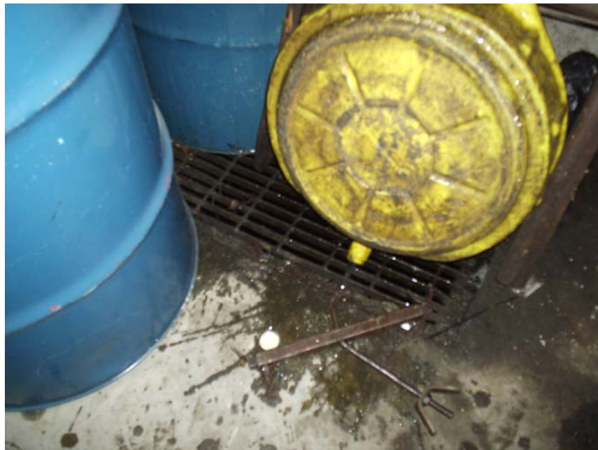
Photograph 6: Interior Drain and Oil Staining
