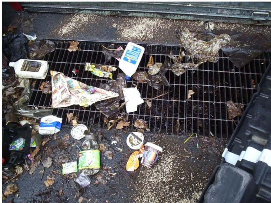
Photograph 8: Trench Drain with Heavy Oil Staining
