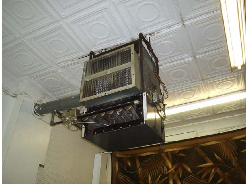
Photograph 5: Overhead Natural Gas Fired Heating Equipment, Typical
