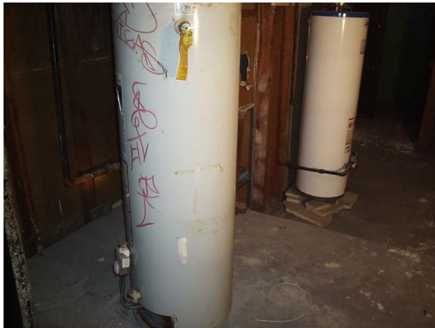
Photograph 6: Natural Gas Fired Hot Water Heating Equipment, Typical
