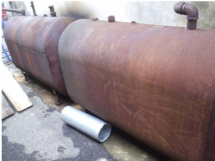
Photograph 8: Aboveground Fuel Oil Storage Tanks
