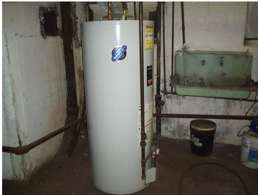
Photograph 7: Natural gas Fired Hot Water Heating Equipment
